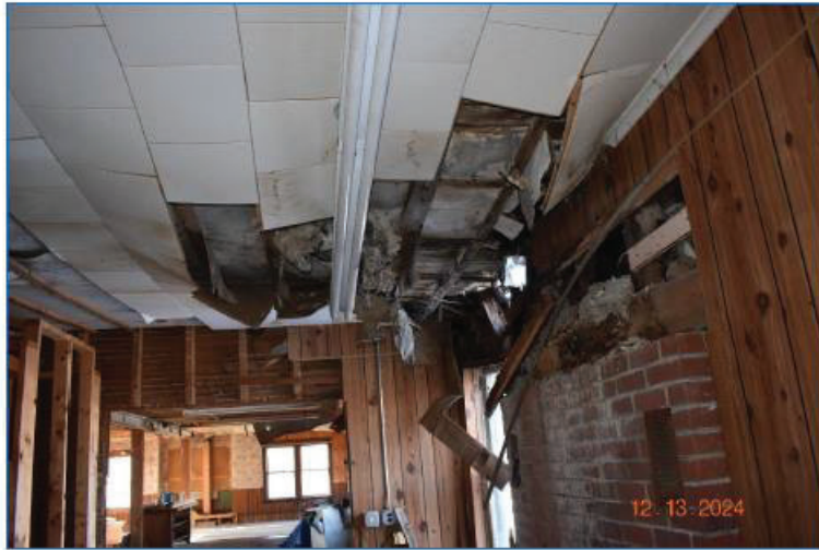
The roof ceiling collapsed near fireplace.
