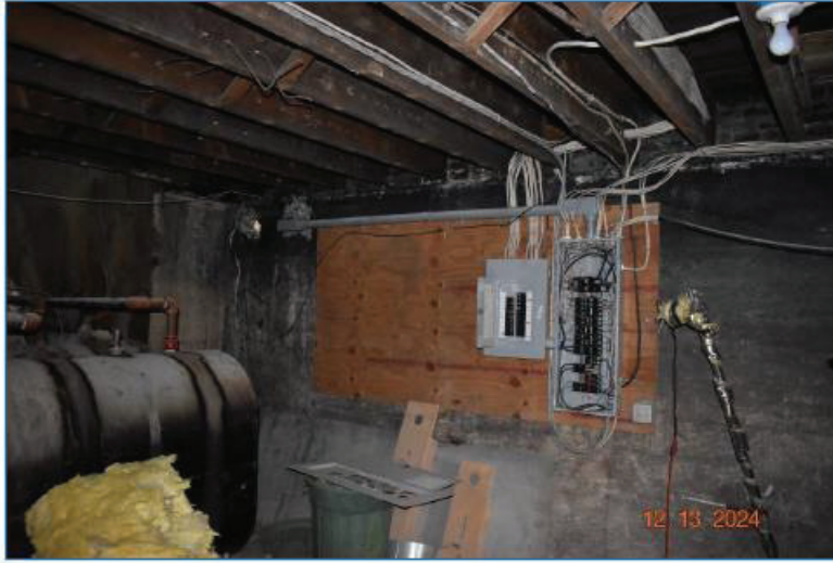
Electrical Entrance and oil tanks (2)
