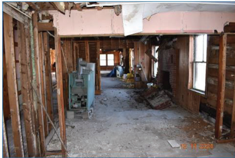
Looking westerly along the north wall. Note the mantel fallen from the brick fireplace.
