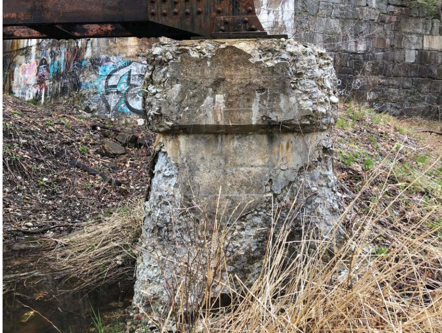
Photo 3. View of southern bent footing showing extents of deterioration and spalling. MaineDOT, April 28, 2020
