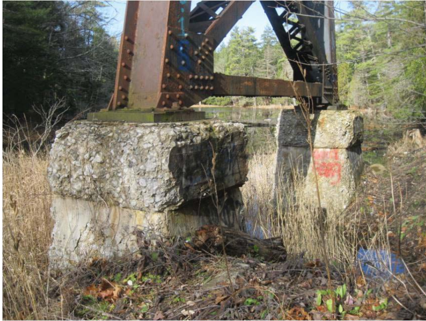
Photo 1. View of the deteriorating bent pier footings of Bridge #7647, Sewall's Creek in Bath. MaineDOT, November 25, 2019
