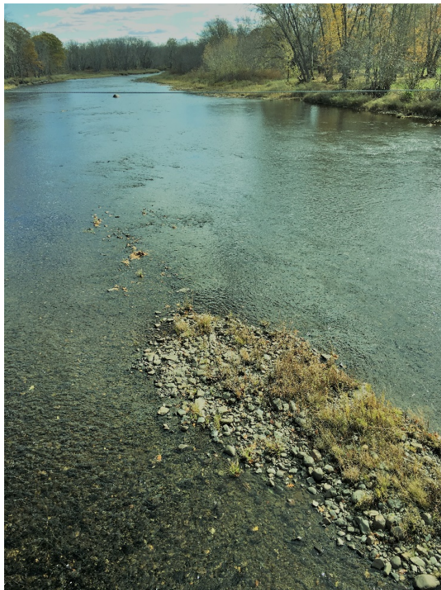
Top: view upstream from west bank; Bottom: view downstream showing river substrate and mid-stream bar in lee of center pier
