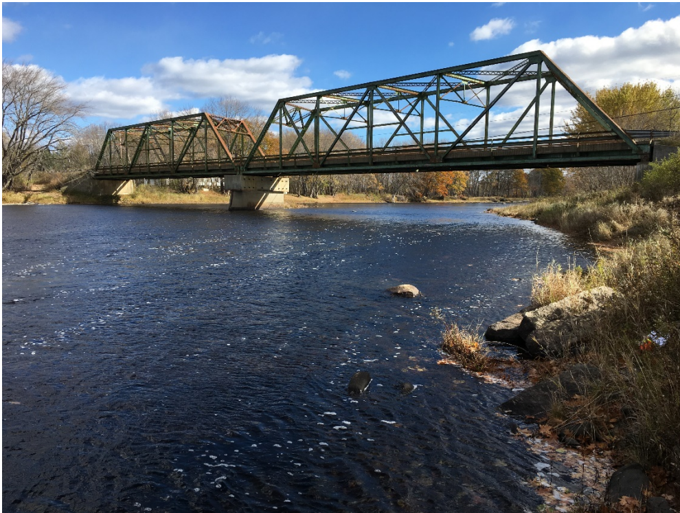
Top: view upstream of bridge from east bank; Bottom: view downstream of bridge from west bank
