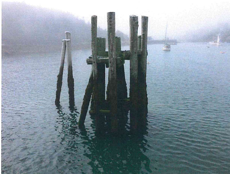
Photo 6. View of timber dolphin (to be removed/upgraded) on the seaward end of the southern side of ferry slip, facing south. MaineDOT, August 2018.
