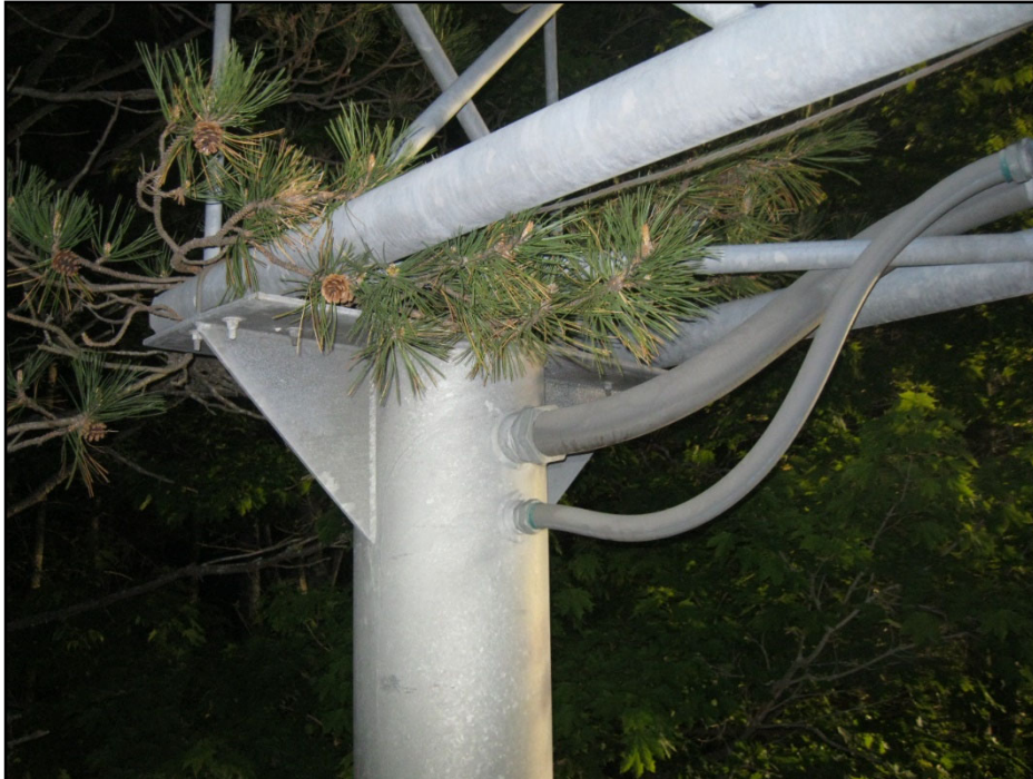
15 Tree encroaching top of west tower, looking northwest.
