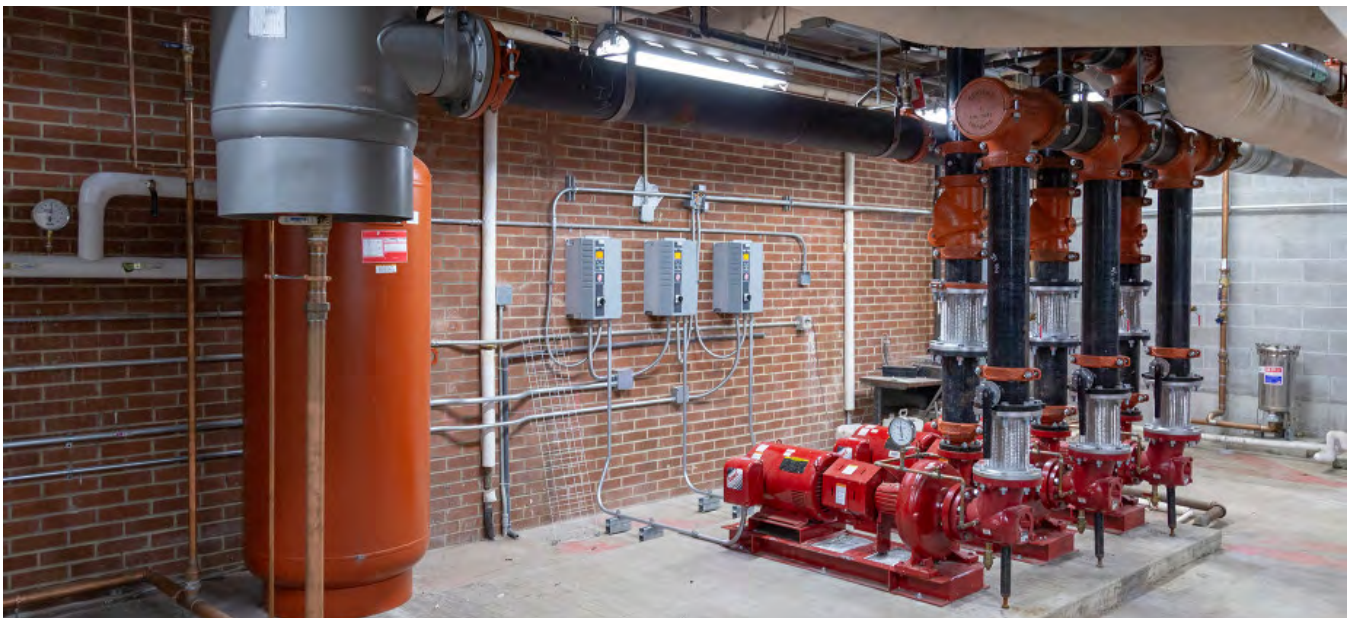
Interior mechanical room with ground-source heat pumps. Courtesy of CMTA, Inc.
