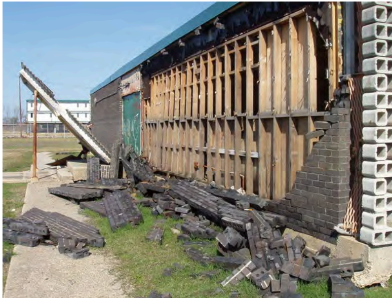
Helen S. Edwards Elementary School, New Orleans after a hurricane
