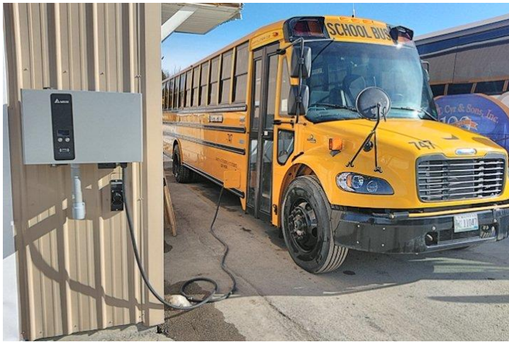
2 Electric bus and charging station
