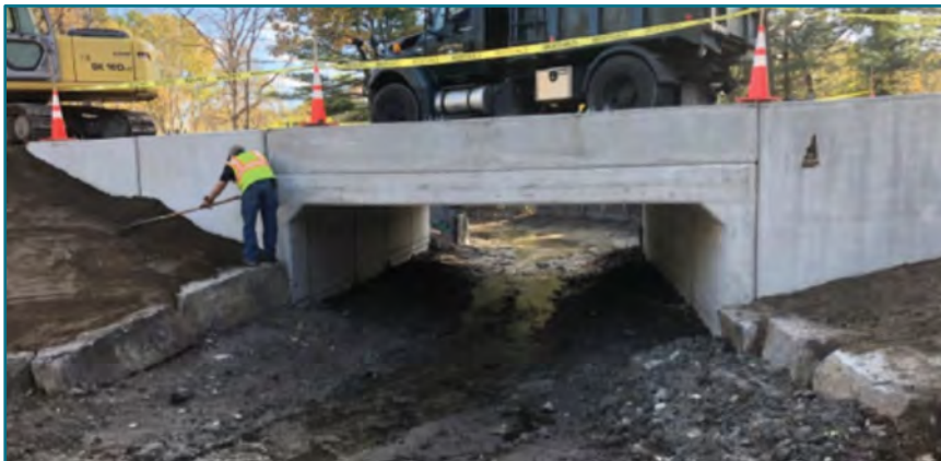
FIGURE B.5 - An embedded pre-cast concrete box culvert, with 16-foot span by 8.5-foot rise. Lubberland Creek, Newmarket, NH. Image source: Peter Steckler.
