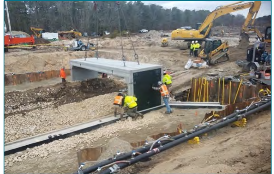
FIGURE B.10 - A three-sided rigid frame section being installed on pre-cast footings. Coonamessett River, Falmouth, MA. Image source: Betsy Gladfelter.
