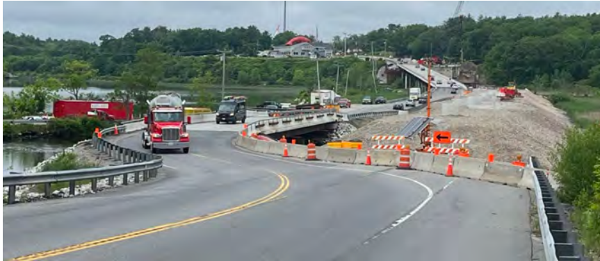
FIGURE 8.1 - When tidal crossings are replaced in primary traffic corridors, temporary traffic bypasses may be required. This temporary bypass along Route 1 in Woolwich, Maine, was used during bridge replacement and construction to restore tidal flow to Back River Creek Marsh. Photo by Michael Burke.
