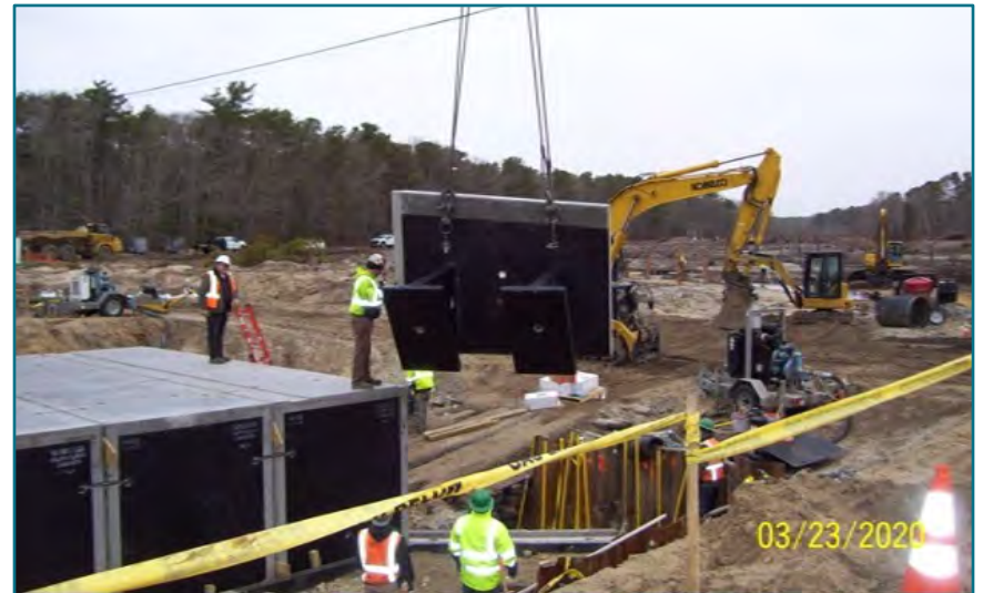
FIGURE B.11 - A pre-cast wingwall installation for a three-sided rigid frame with pre-cast footings. Coonamessett River, Falmouth, MA. Image source: Chris Bennett.
