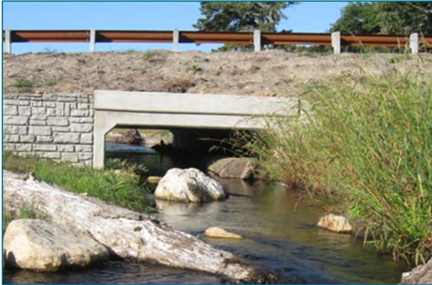
FIGURE B.4 - A reinforced concrete box structure with prefabricated wingwalls and an installed channel bed. Structure size in this example was five feet rise by ten feet span. Eel River, Plymouth, MA. Image source: Inter-Fluve.
