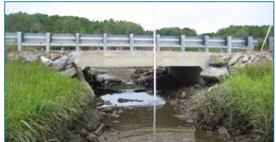
FIGURE B.7 - A three-sided concrete rigid frame structure, installed on Wallace Shore Road (private) in Harpswell, ME. Image source: Matt Craig.
