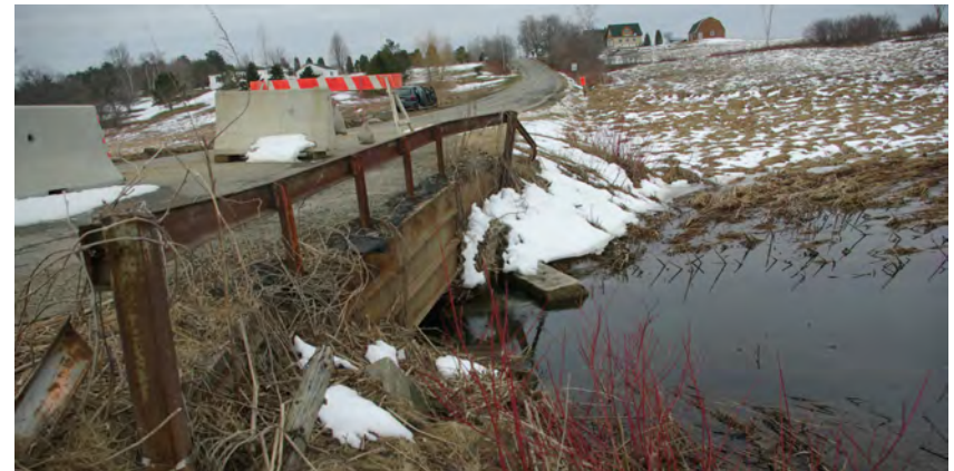
FIGURE 1.14 - Like many aging crossings, this one was replaced well after its safe, useful service life concluded. Photo by Slade Moore.
