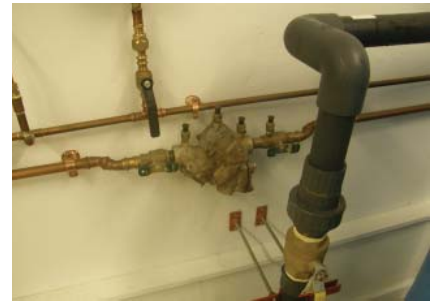
A testable backflow prevention device on a treatment feed line
