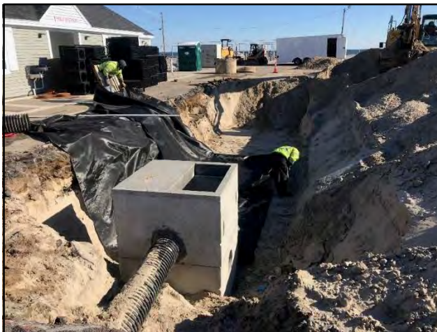
Installation of enhanced drywell and catch basin inserts to treat the runoff from the Main Beach Parking Lot.
