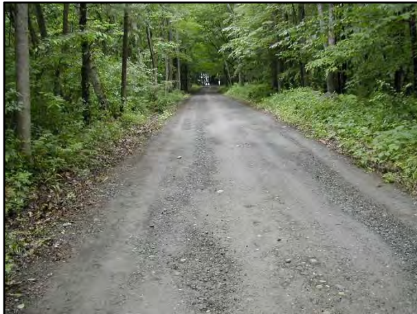
Before - Upper section of Ware Road showing surface erosion prior to improvements.
