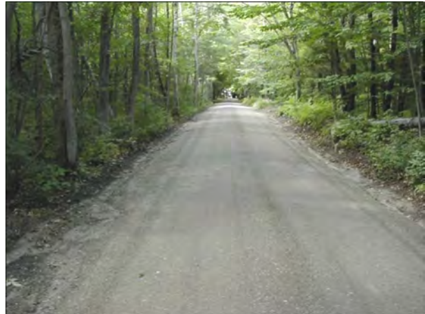
After - Same section of road with new surface gravel, crowning, and grader berms removed.
