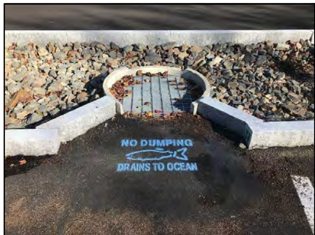
Stenciled catchbasin draining to the Leavitt Stream tributary to the Ogunquit River.
