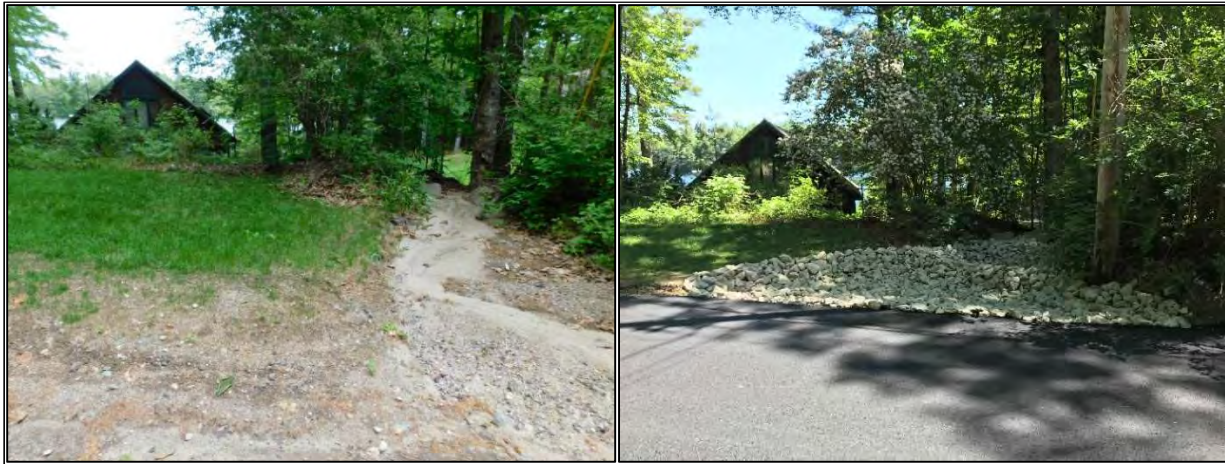
Prior to the Phase II project, Lakeside Drive experienced chronic erosion with direct flow into the lake (above left). Numerous BMPs were installed to stabilize the road surface including 900' of road grading and paving, riprap ditches, turnouts, and a detention basin with level spreader (above right).
