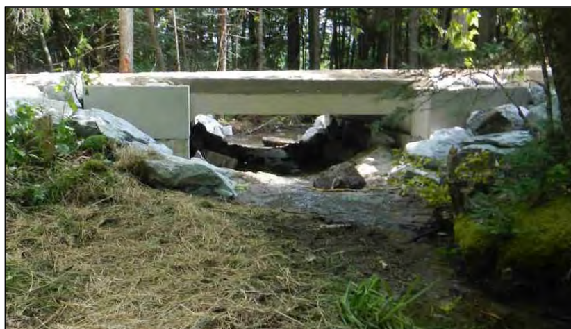
The Fitts Mountain Road stream crossing in Dedham was replaced with combined funding from a Stream Crossing Grant ($20,000) and CWA Section 319 ($8,665) as part of Hancock County SWCD’s Phillips Lake Watershed Protection Phase II Project.
