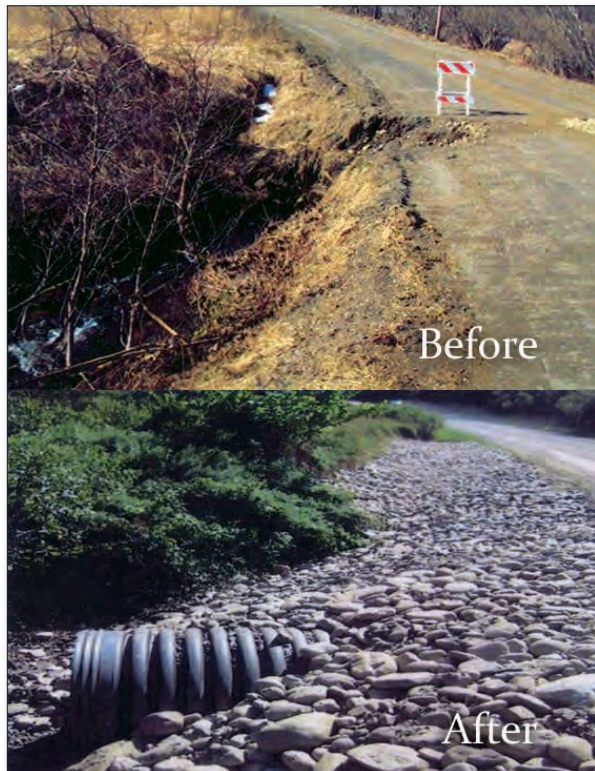
Figure 2. Marden Hill Road, before (top) and after (bottom) completion of an erosion control project.
