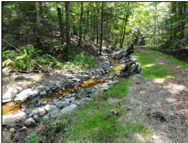
After - Lower reach stabilized with pool and cascade structures, riffles, and rock veins.
