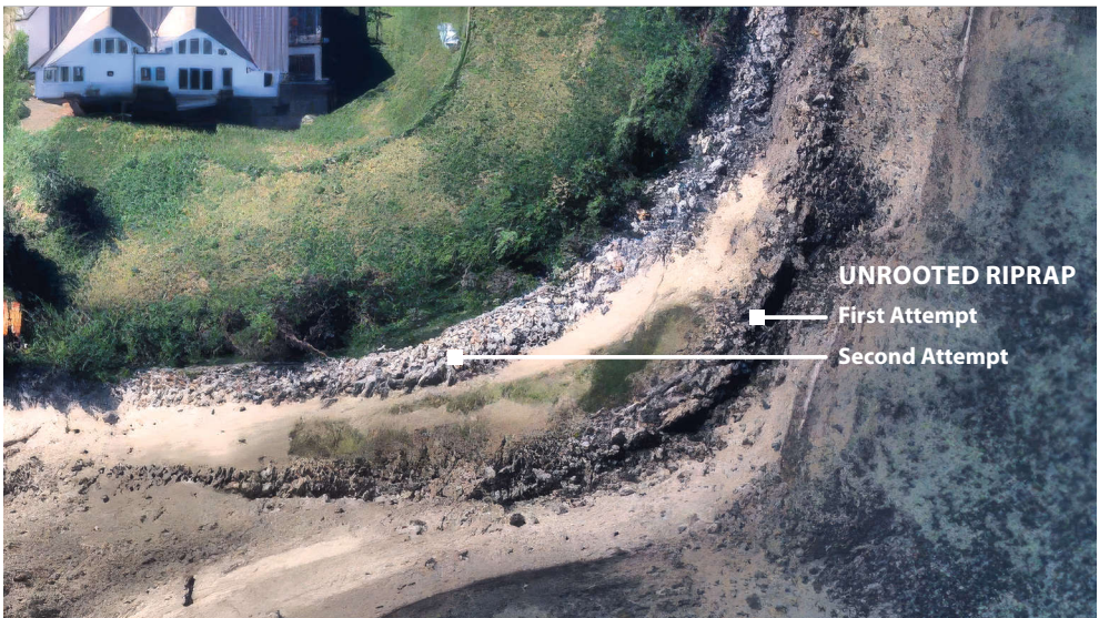
Unrooted riprap was installed twice in front of this house. It failed both times to prevent erosion.
