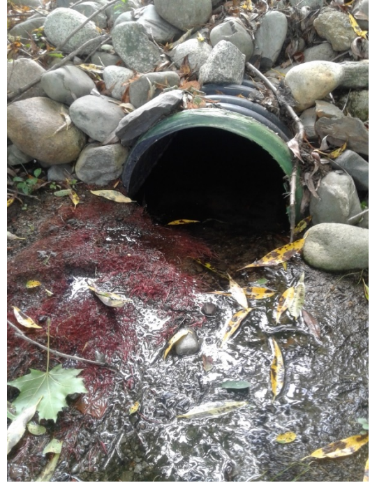
Fig. 2. This outfall is partially submerged and a clean catch of its discharge is not possible.
