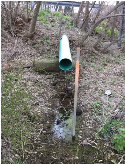
This outfall, though in poor condition because it is cantilevered, provides a good opportunity for a clean catch of its discharge.
