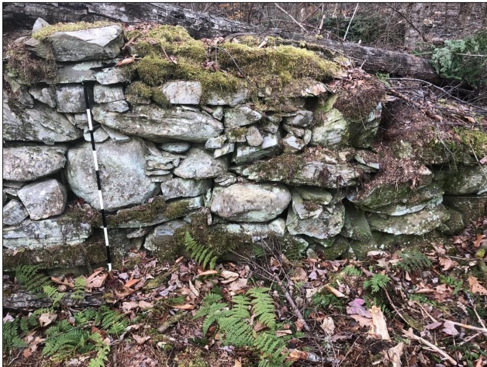
Figure 5-59. East half of intact south wall of structure at Site ME 441-005, facing north.
