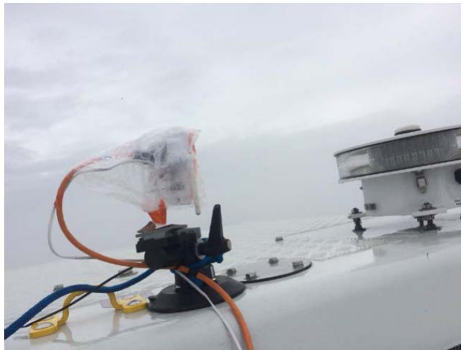
Figure 18. Webcam Used to Monitor Obstruction Light Status During Assessment [7]
