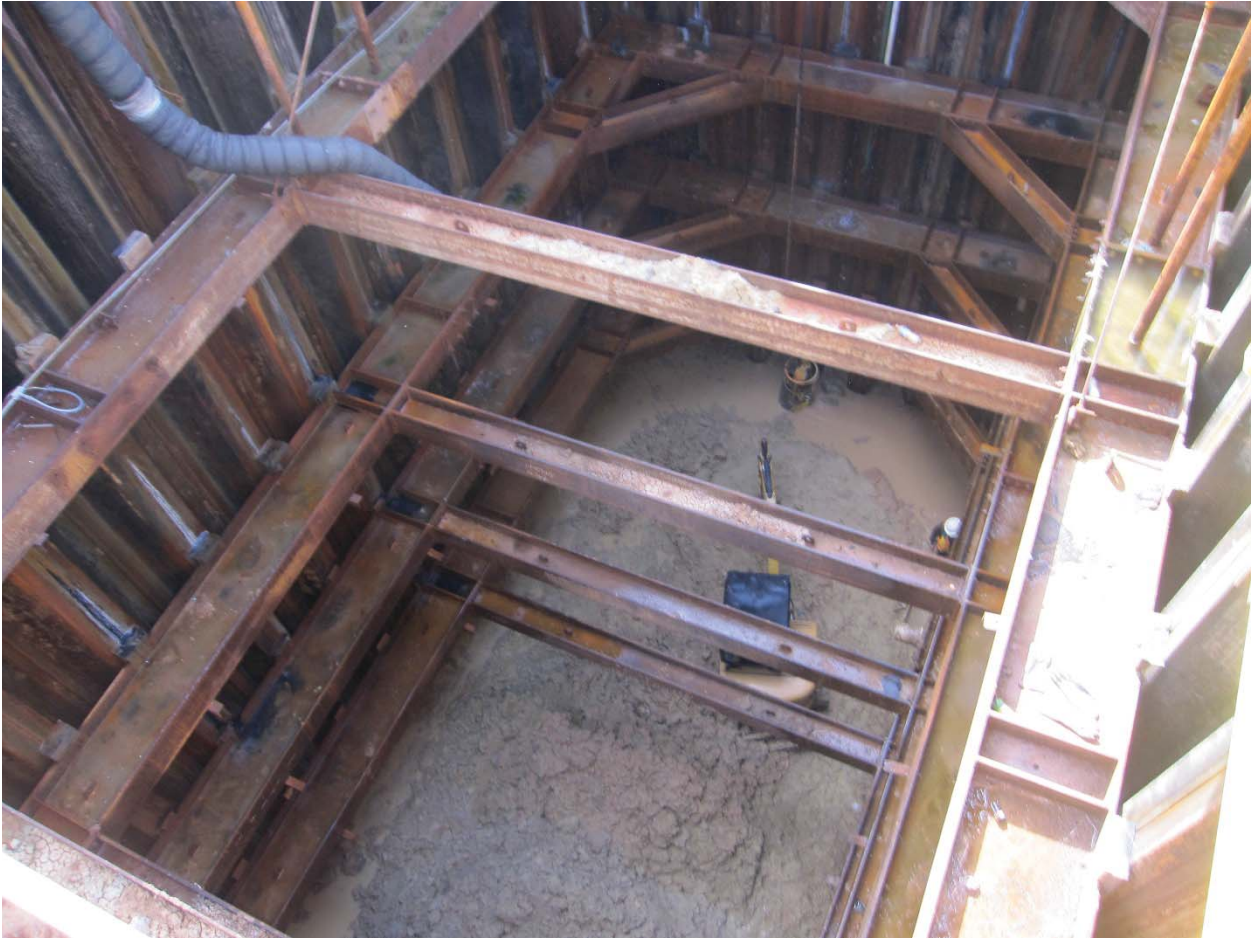
Example of a narrow sheet pile structure with struts to suit this type of work.
