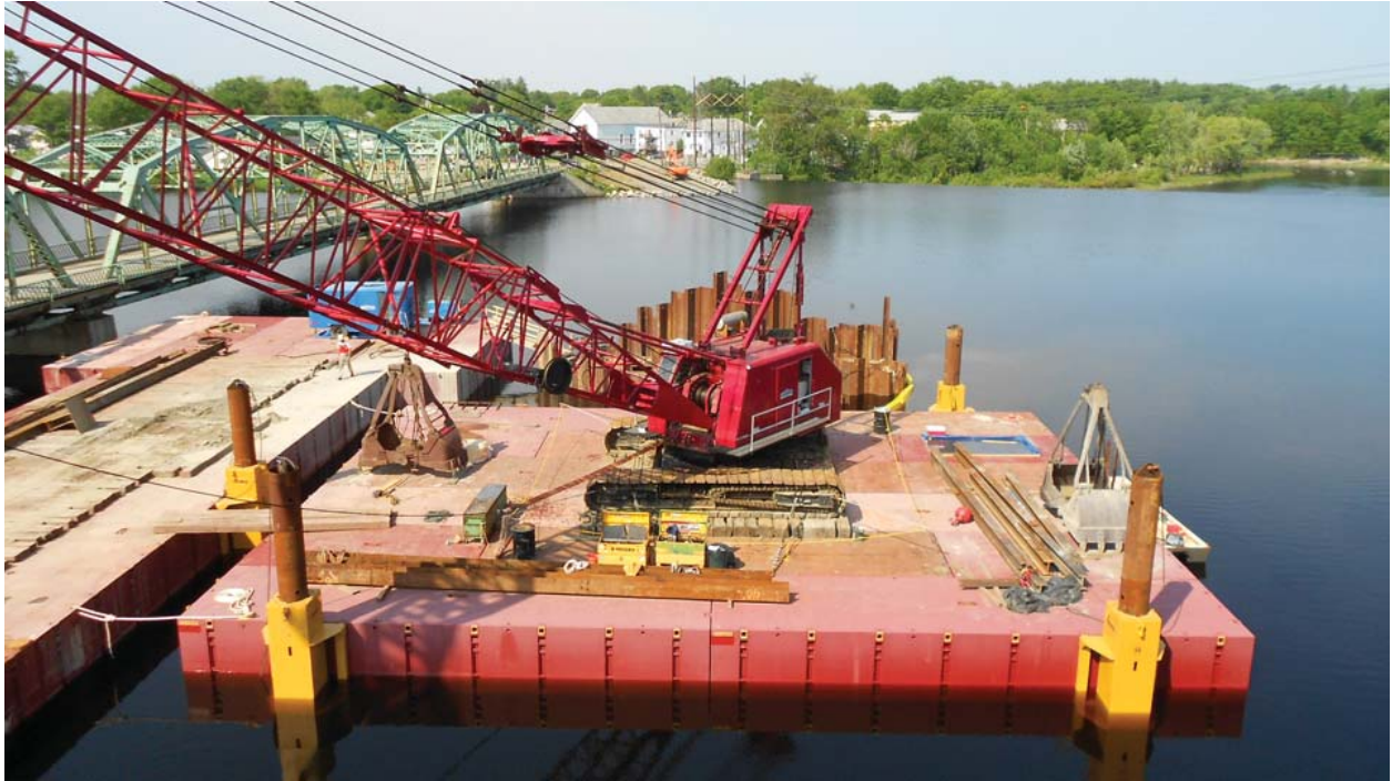
Example of a spud barge with crane, clamshell suited for this work.
