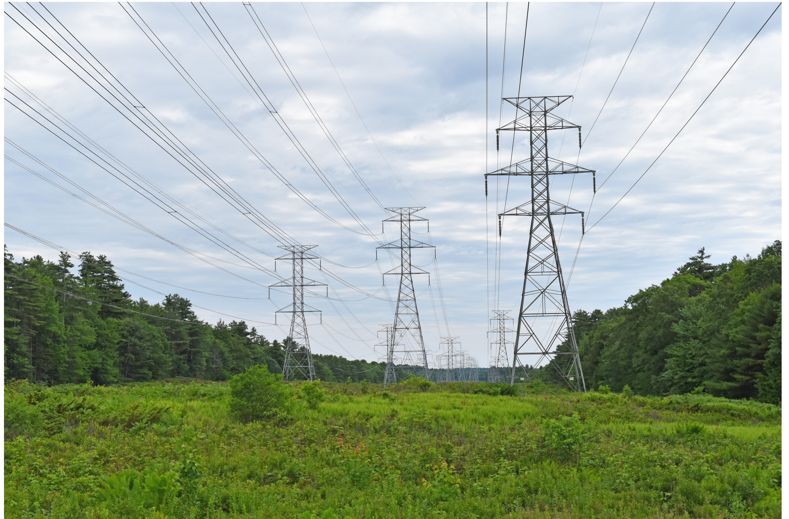
Proposed Conditions: Normal view looking south from Route One in Wiscasset toward the proposed co-located 345 kV transmission line. The only visible change will be the new conductors added to the middle lattice structure.
