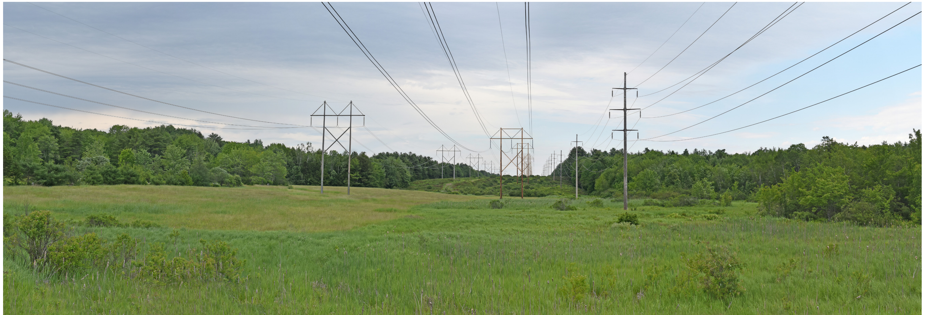
Proposed Conditions: Panoramic view looking from north to northeast from Route 27 toward the proposed co-located 345 kV transmission line. The proposed 345 kV transmission line will be located in between the existing 115 kV and 345 kV transmission lines. A proposed structure will be located directly adjacent to this viewpoint. Seven structures and conductors will be visible from this viewpoint. See Appendix B: Study Area Photographs for additional images.
