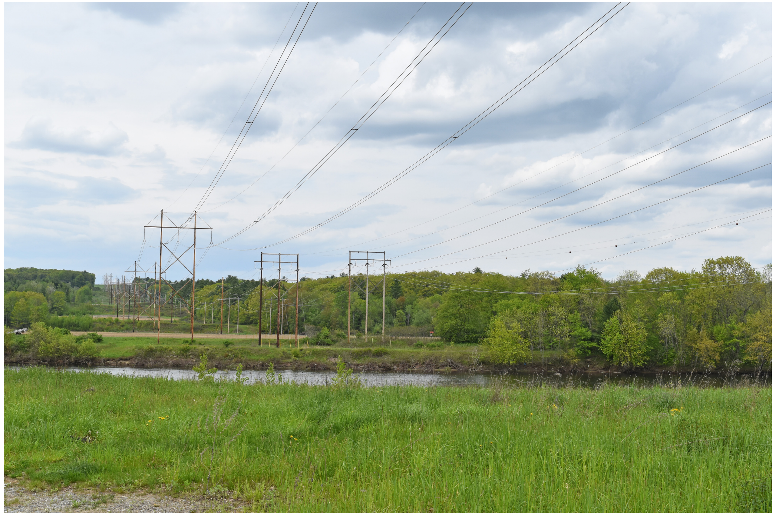
Existing Conditions: Normal view looking from northeast from Riverside Road / Route 136 in Auburn over the Androscoggin River toward the existing 115 kV and 345 kV transmission lines.
