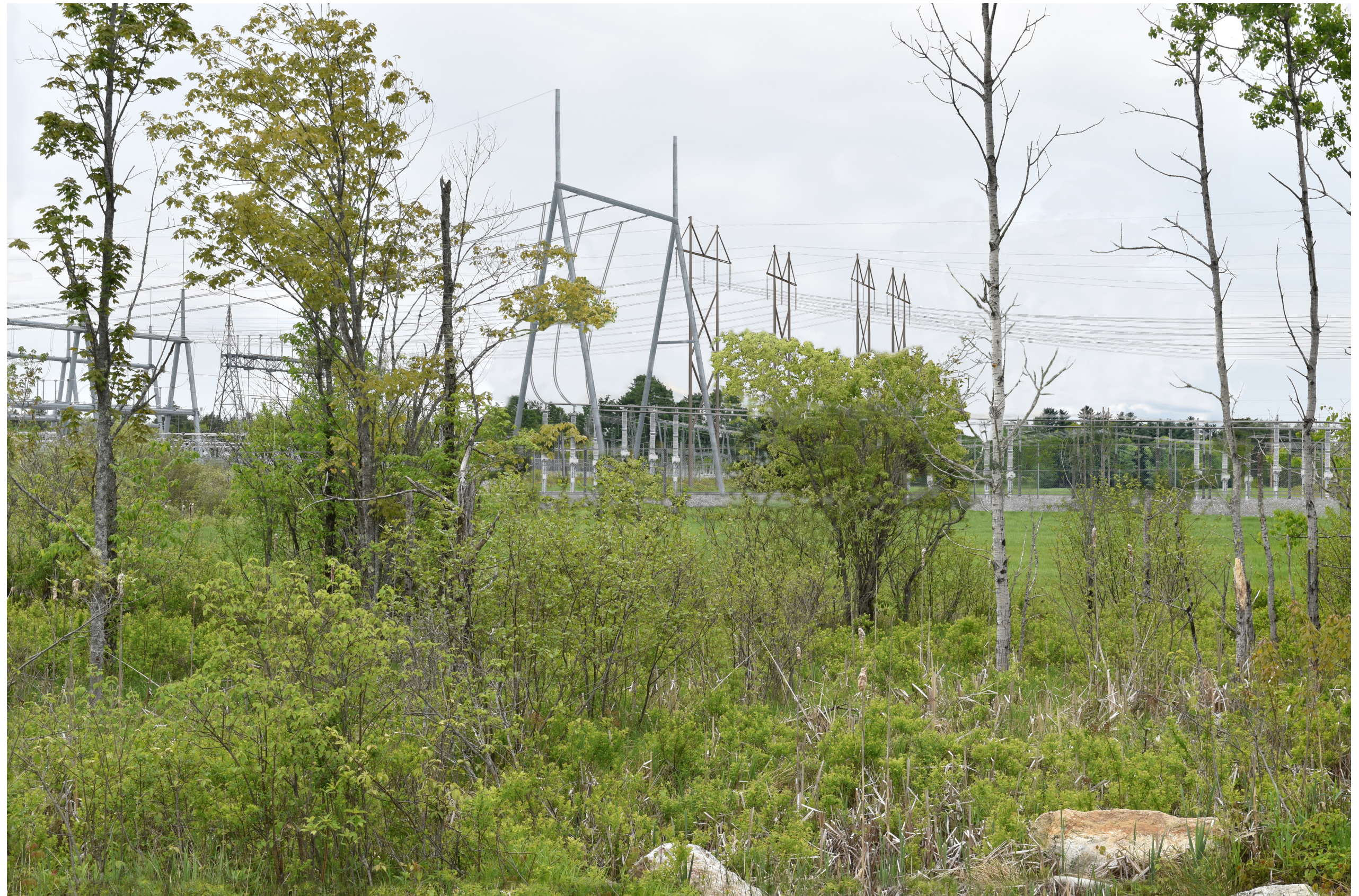
Proposed Conditions: Normal view looking south from Fickett Road toward the proposed Fickett Road Substation and the Sections 62 & 64 Rebuild transmission lines. The visible substation components will range in height from 15' to 60' and will be silver gray in color. The closest substation components will be 450 +/- feet from Fickett Road. Other visible components will include the enclosure fence. The evergreen trees in the middle of the field will be removed.
