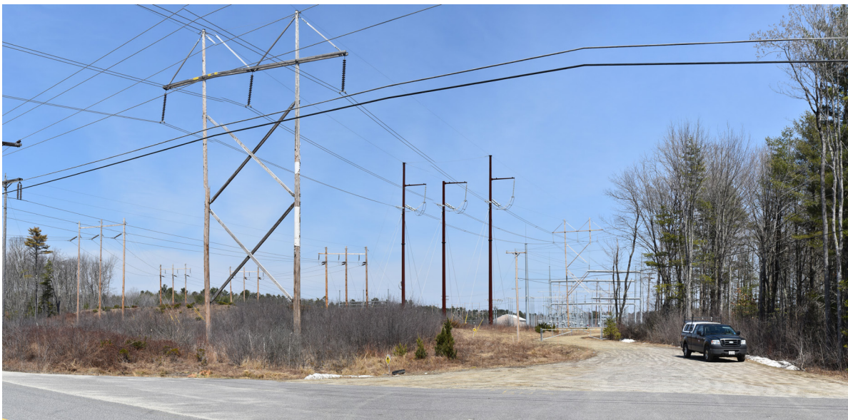
Viewpoint 2: View looking northeast toward Raven Farm Substation in Cumberland. The components of the substation expansion will be minimally visible where the access road meets Greely Road. The partially visible components will be seen to the left of the tan sided building in image and behind the three self weathering steel single poles in the center of the image. The proposed components will be the same size and color as existing components and partially screened by the existing earth berm and buffer plantings.
