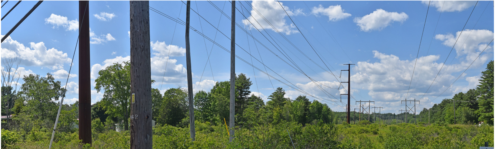
P9-8: Panoramic view looking north toward the Rebuild Sections 64 at the Sabattus Street crossing, Lewiston. The 115 kV transmission line on H-frame structures will be rebuilt onto to single pole wooden structures. No additional tree removal is required.
