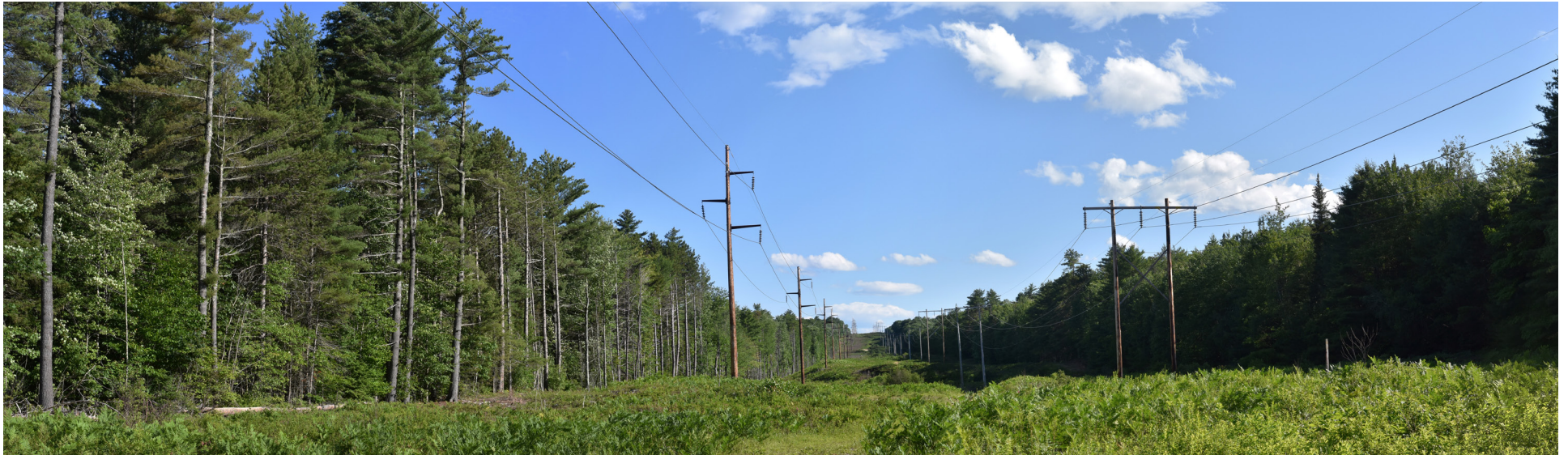
P8-15: Panoramic view looking south down the existing 115 kV transmission corridor where it crosses the portion of Androskoggin Riverlands that is east of the river in Leeds. The existing 150' wide transmission line corridor will be widened by 75' on the western side to accommodate the proposed HVDC transmission line.
