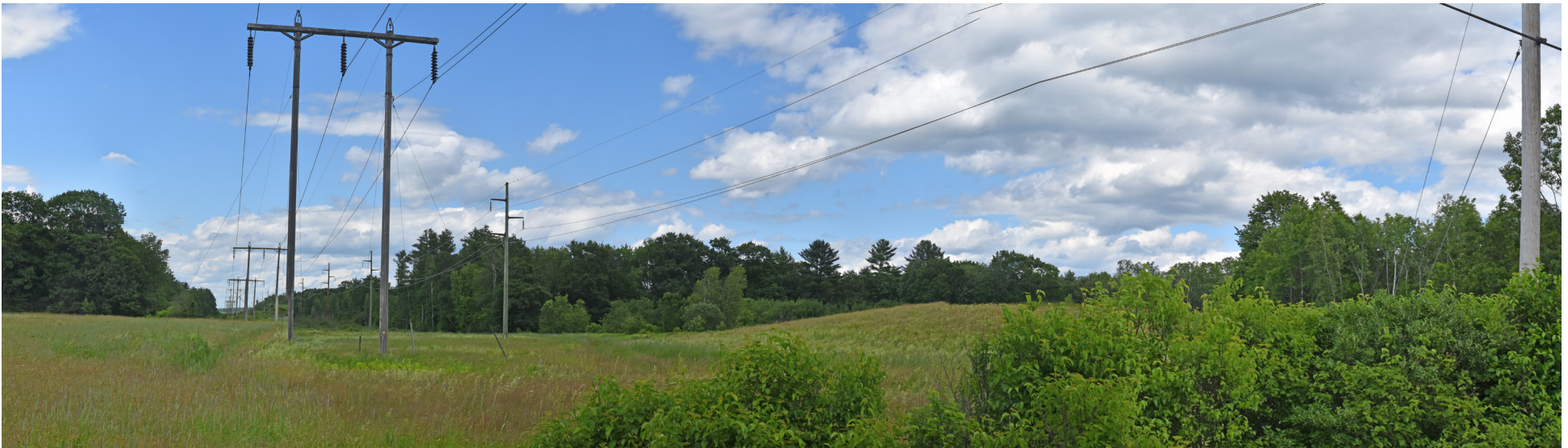
P8-10: Panoramic view looking north at the existing 115 kV transmission corridor from the Strickland Loop Road crossing in Livermore Falls. The existing 150' wide transmission line corridor will be widened by 75' on the western side to accommodate the proposed HVDC transmission line.
