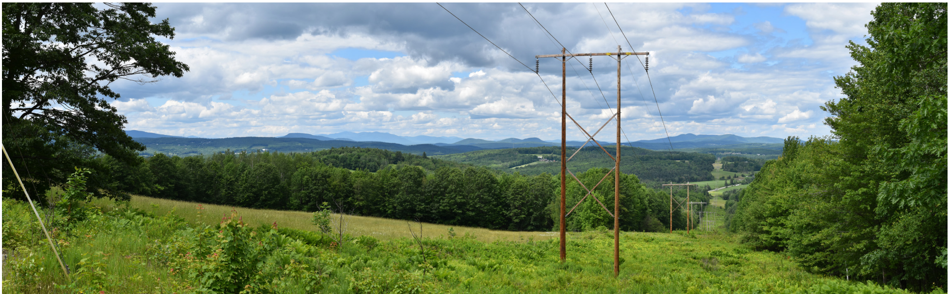
P7-14: Panoramic view looking northeast down the existing 115 kV transmission corridor from the Soules Hill Road Crossing in Jay. The existing 150' wide transmission line corridor will be widened by 75' on the west side to accommodate the proposed HVDC transmission line.
