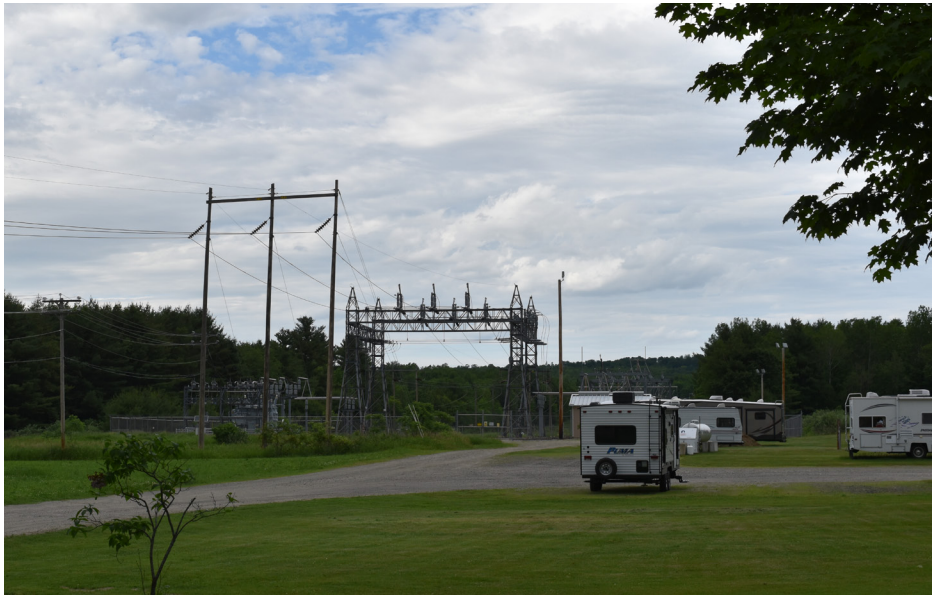
P7-12: View looking north at Sturtevant Substation near the Route 2 crossing in Farmington. See Photosimulation in Appendix D for view in opposite direction.
