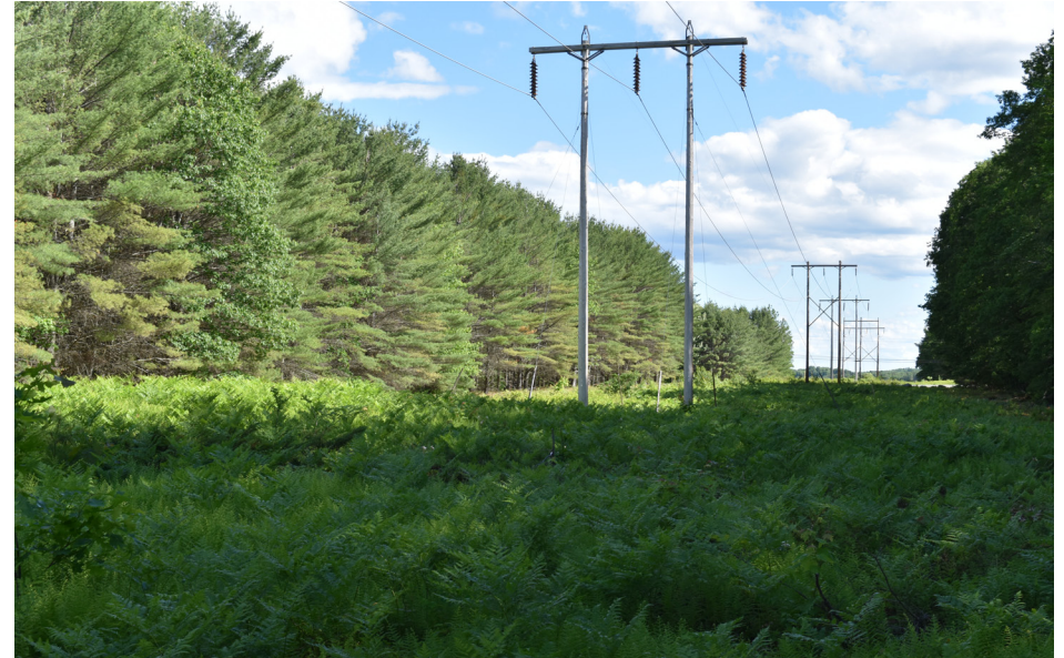
P5-18: View looking north of existing transmission line where it crosses the Kennebec Valley Trail. See Photosimulation from Route 8 in Appendix D.
