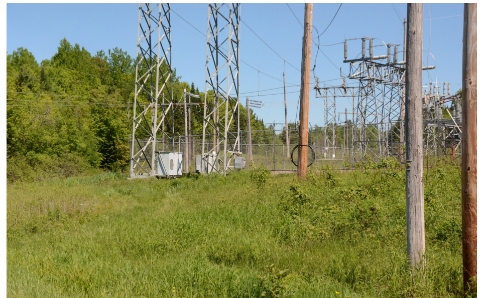
P5-10: Looking north toward the existing substation off Bert Berry Road in Embden.
