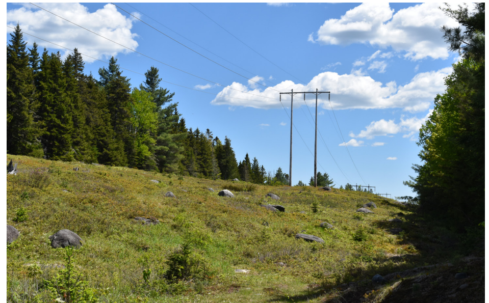
P4-3: Existing transmission line corridor crossing near intersection of Baker Dimmock Road and Trestle Road.
