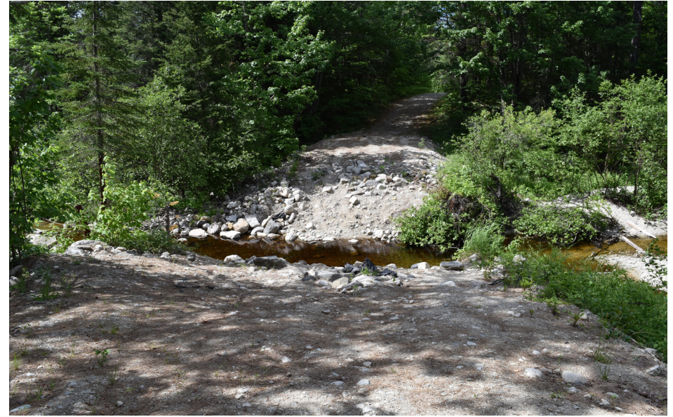
P2-5: The Spencer Rips Road is currently not accessible to vehicles from Spencer Road because the bridge was removed. Repairs proposed Sept. 2017.
