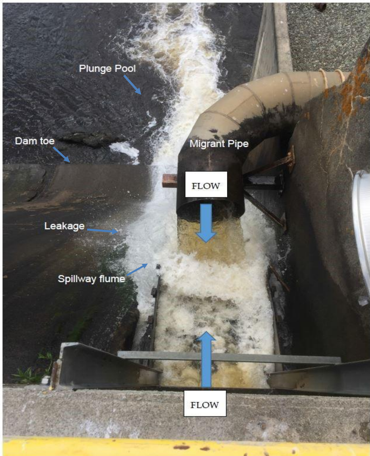
Figure 17. Downstream fish passage facility spillway flume at Ellsworth Dam. (Source: Black Bear Hydro, 2015b, as modified by staff).
