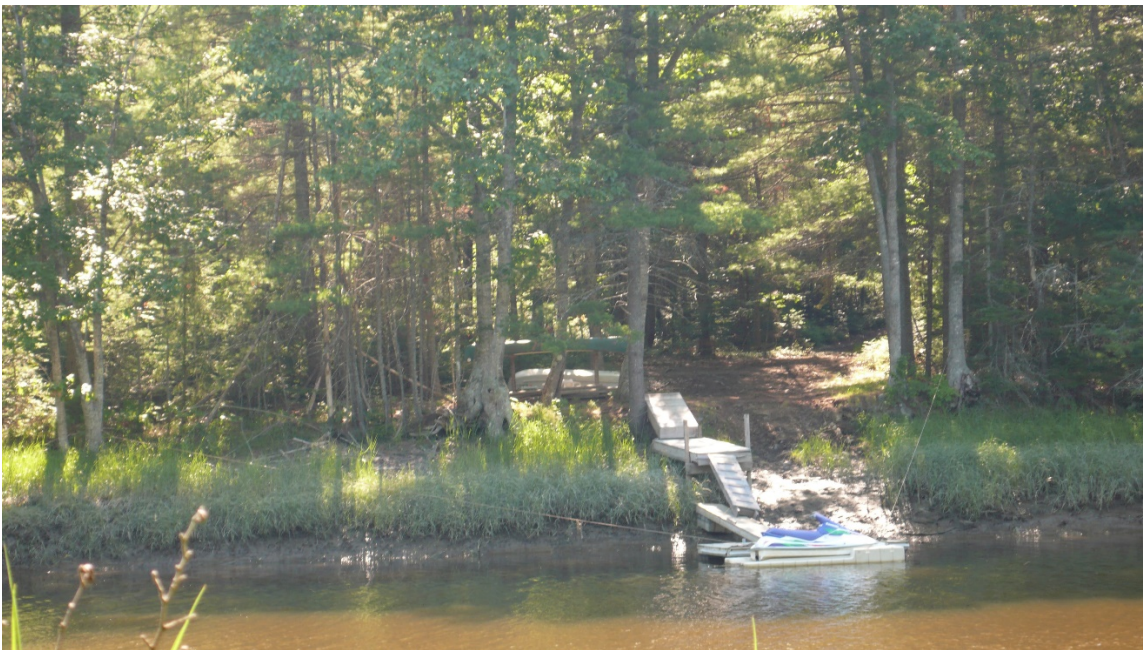
July 13, 2007: The first dock installation now is complete, four years after issuance of permit. Note short extension over the riverbank, narrow width of actual dock-plank, all of wood, no railings. For comparison purposes later, check the size of the clearing. Although still permanent, the size is small.
