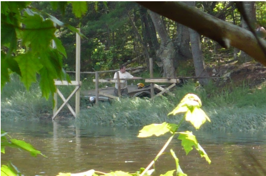
Figure 1. June 24, 2012 photo of Jeff Spinney in the process of constructing a permanent pier. Noteworthy is that even as the permanent pier was being constructed, water was already at or above the pilings closest to the river, despite the likelihood that this photo was not taken at or near the time of highest annual tide.
