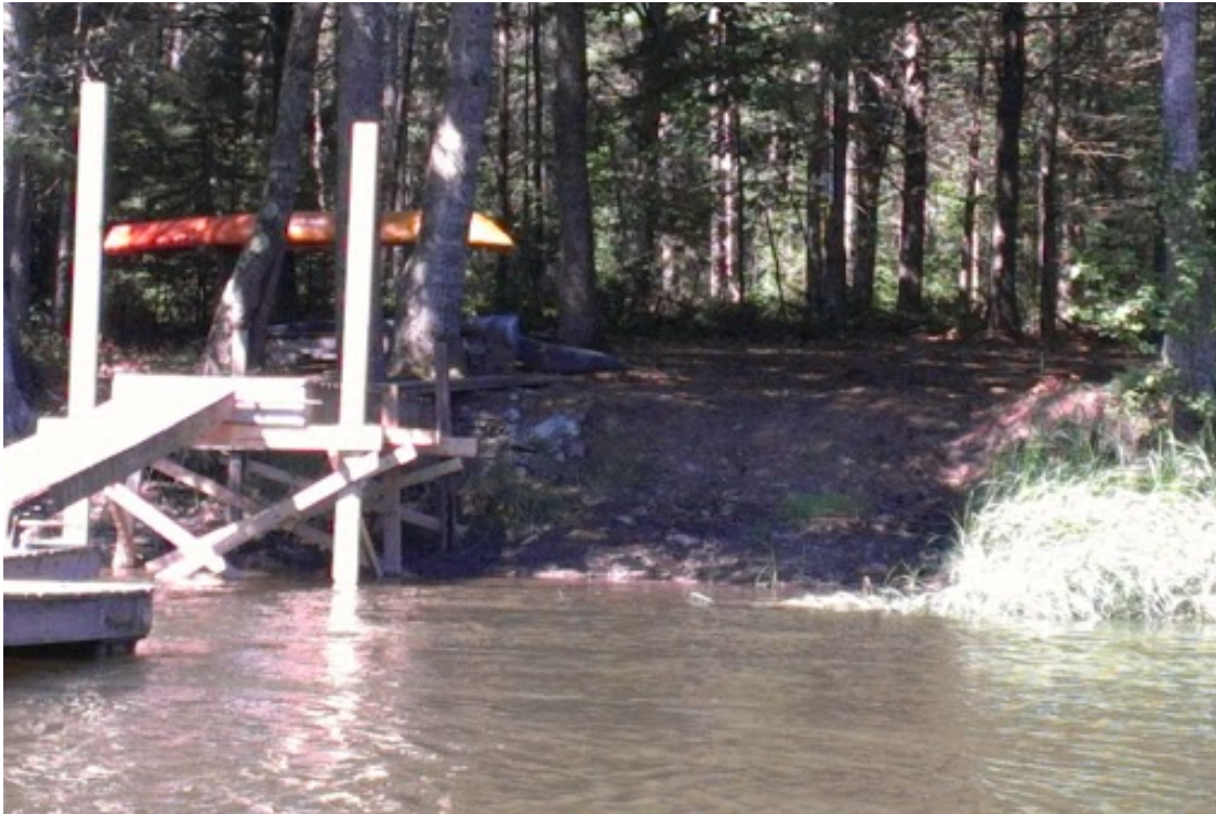
Figure 2. July 31, 2012 photo after completion of Spinney’s permanent pier structure, showing tide level above the second row of permanent pilings.
