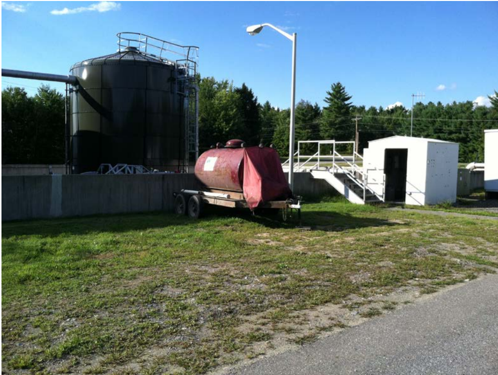
Figure 2. Small Leachate Storage Tank
