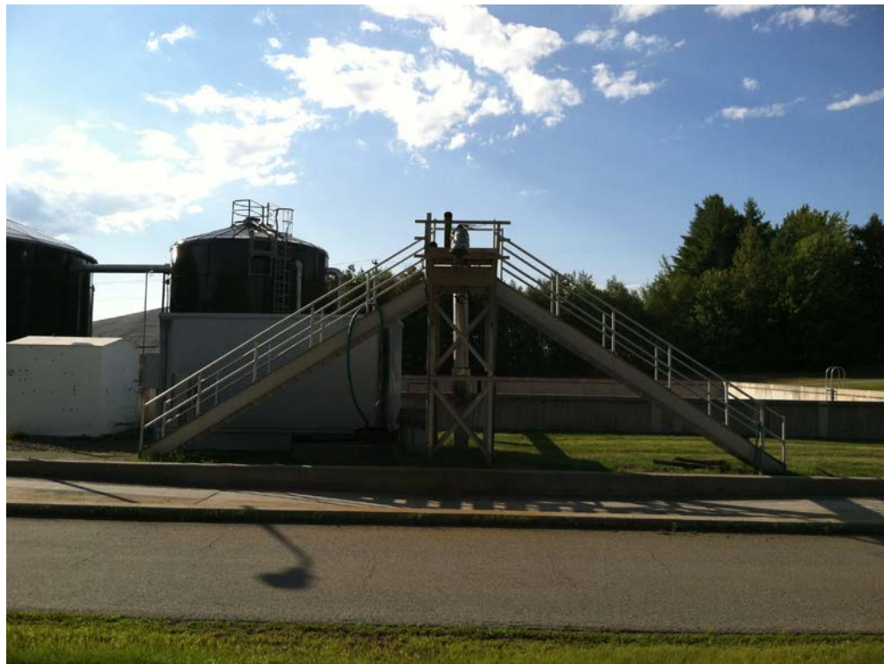
Figure 5. Leachate Load-out Station – Side View
