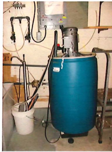
A view of an empty drum that formerly contained sodium hydroxide to be used in the neutralization tank.
