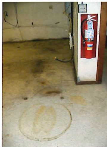
A view of the former location of two cyanide waste drums that were removed by Clean Harbors.
