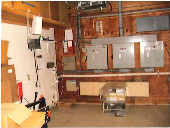
A view of electrical panels and equipment remaining in the Utility Room.
