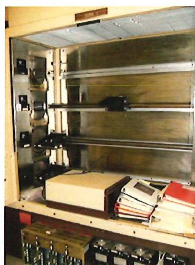
A view of production equipment in the Furnace Room.
