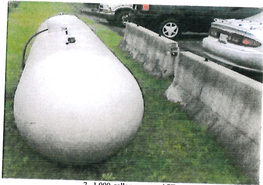
7. 1,000-gallon propane AST.
