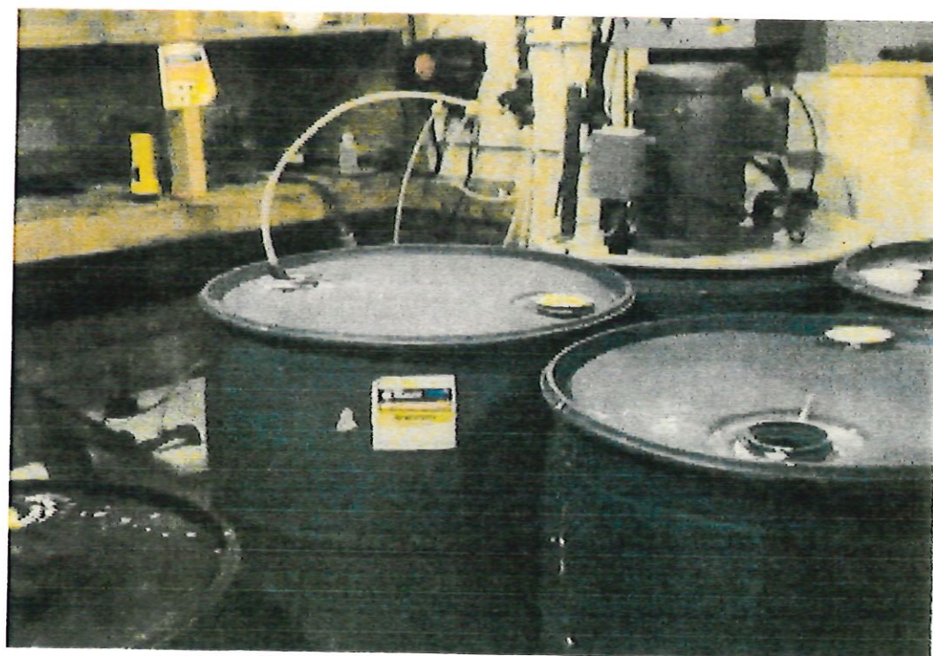
14. Acid neutralization tank area.
