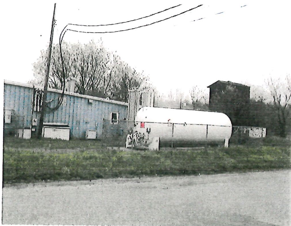
4. 6,000-gallon liquid nitrogen AST. West side of facility.
