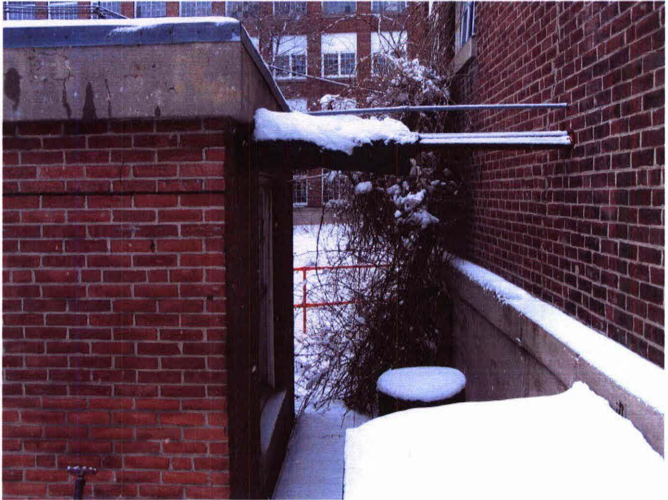
WINTHROP COMMERCE CENTER ASBESTOS INSULATION ON PIPING BETWEEN PUMP HOUSE/BOILER ROOM 1-25-2006 P. BLANCHARD A-157-2005
