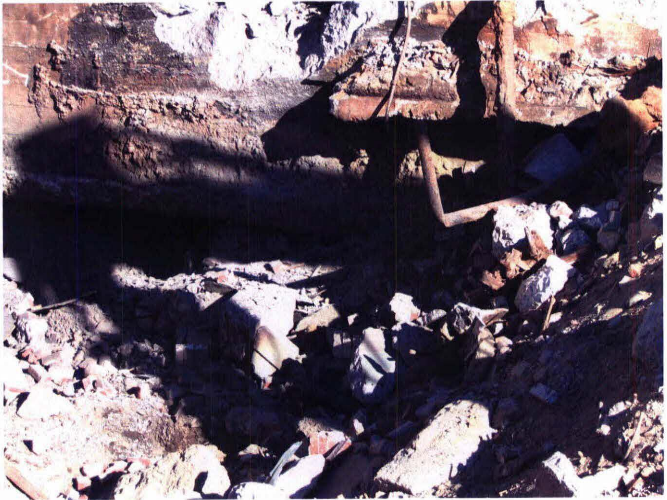
WINTHROP COMMERCE CENTER BOILER ROOM FOUNDATION DEMOLITION PIPING + DEBRIS 3-7-2006 P. BLANKHARD A-157-2005
