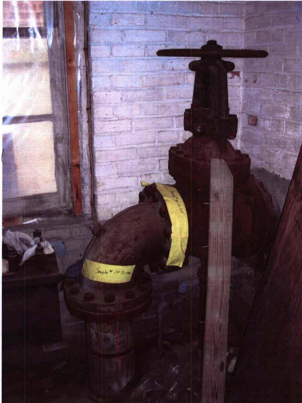
WINTHROP COMMERCE CENTER ASBESTOS GASKETS PUMP HOUSE 1-25-2006 P. BLANCHARD A-157-2005
