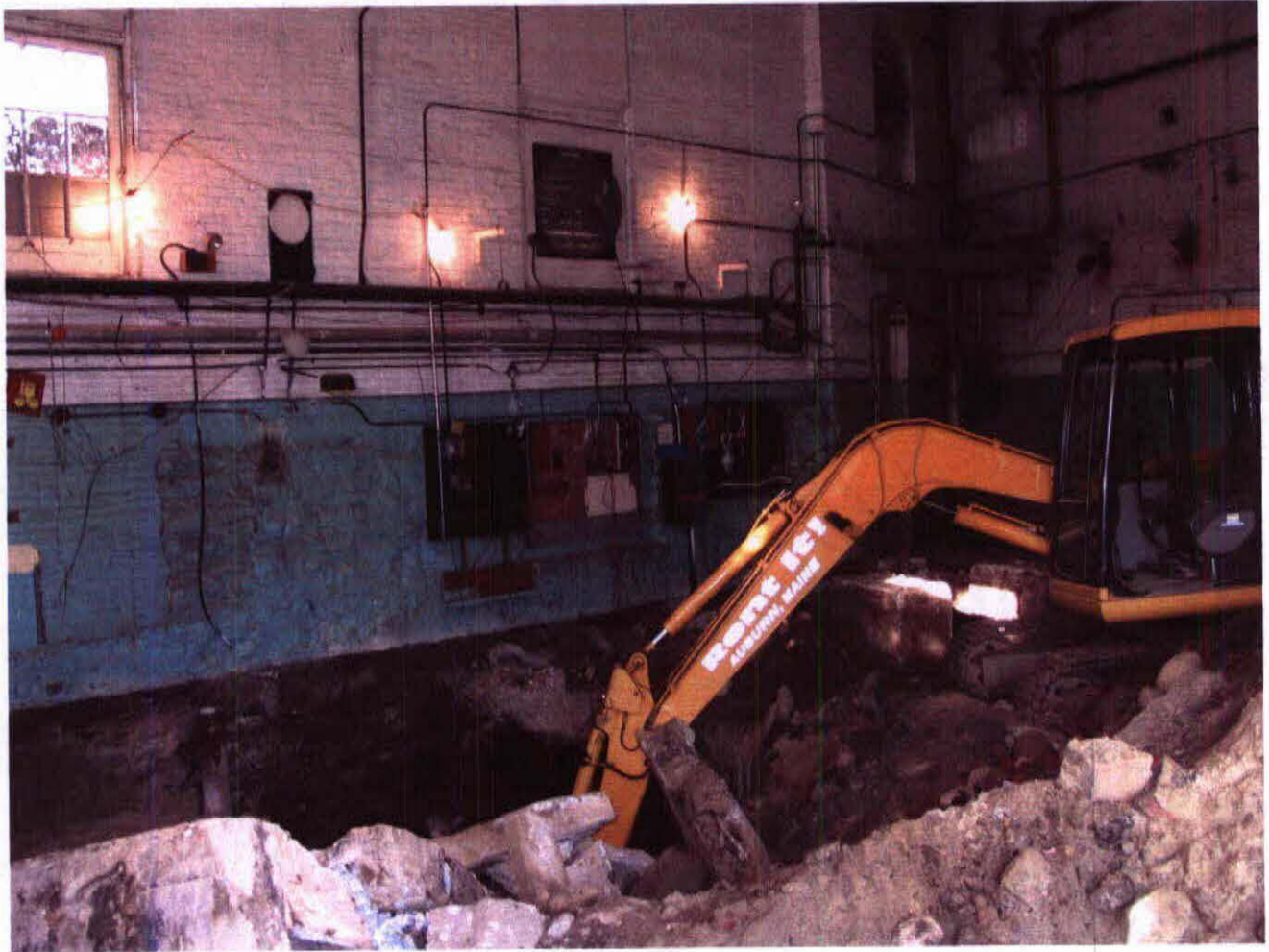
WINTHROP Commerce Center INTERIOR BOILER ROOM 12-1-2005 P. BLANKNARD A-157-2005
