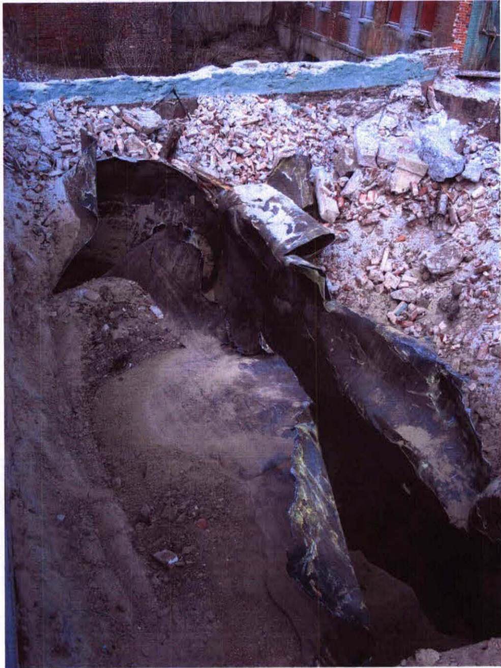
WINTNRUP COMMERCE CENTER UST REMOVAL BY FORCE BOILER ROOM 3-1-2006 P. BLANCHARD A-157-2005
