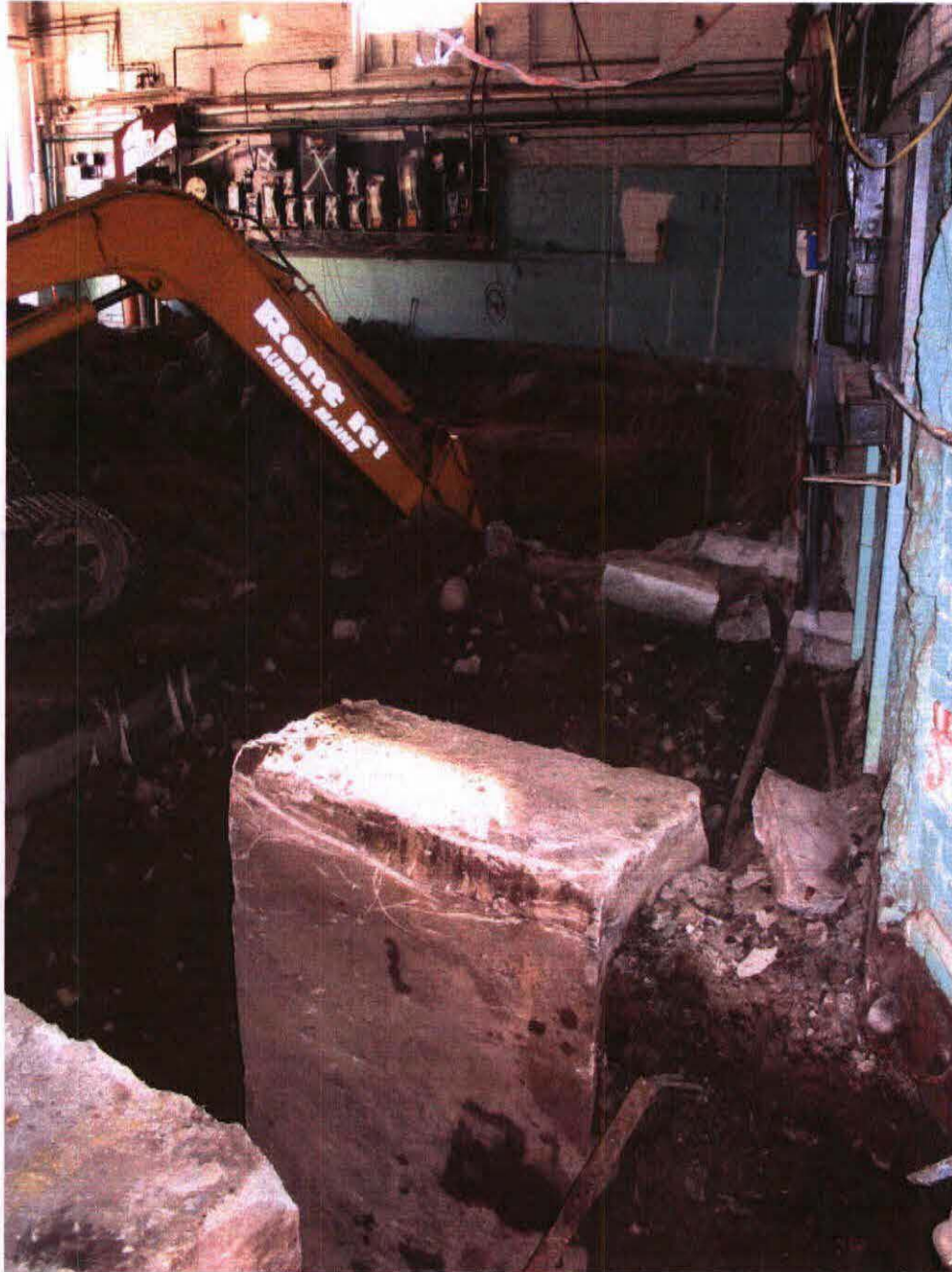
WINTHROP Commerce CENTER INTERIOR BOILER ROOMS UST IN BACKGROUND 12-1-2005 P. BLANCHARD A-157-2005
