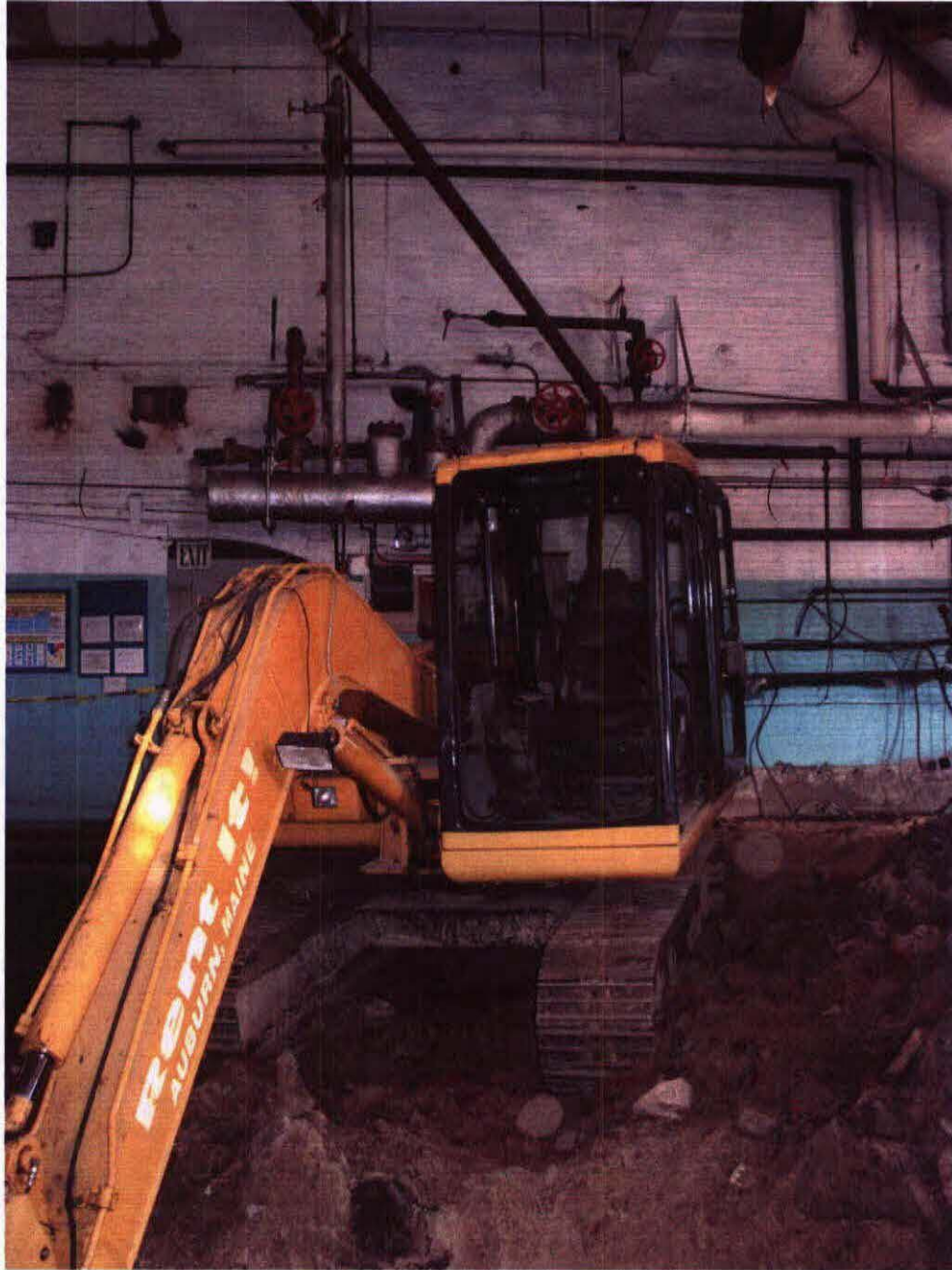
WINTHROP Commerce Center INTERIOR BOILER ROOM 12-1-2005 P. BLANCHARD A-157-2005
