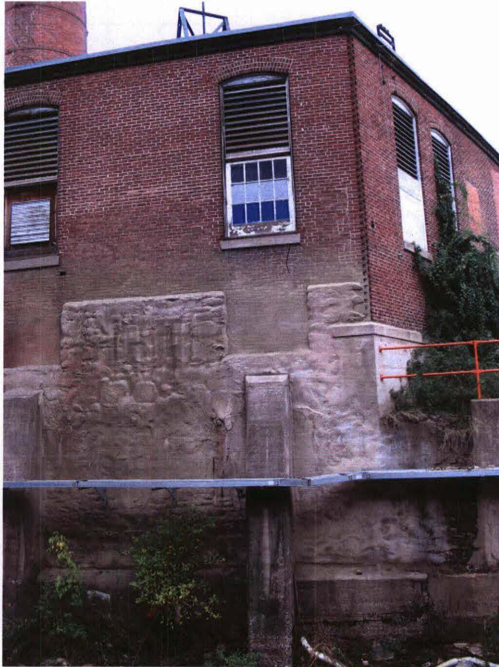
WINTHROP COMMERCE CENTER BOILER ROOM 9-16-05 P. BLANCHARD A-157-2005
