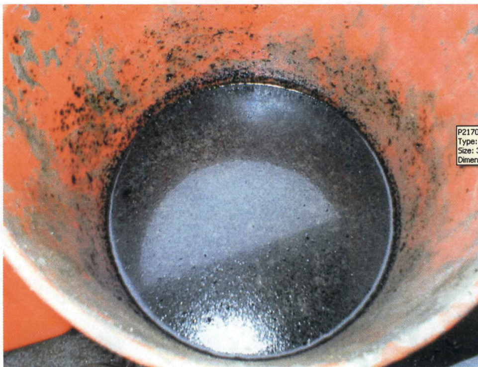
Water and liquid phase petroleum from borings located within the boiler house
