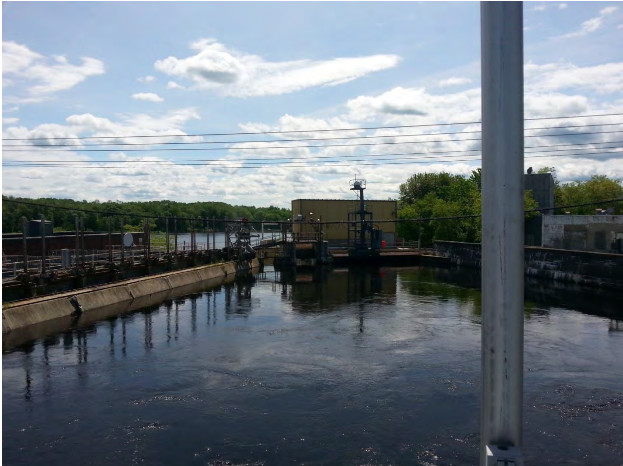
FIGURE 7: VIEW FROM ABOVE THE HEAD GATE STRUCTURE LOOKING DOWNSTREAM INTO THE FOREBAY.
