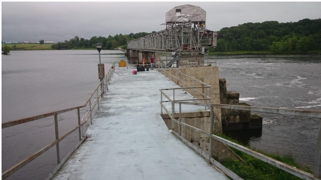
FIGURE 5: VIEW FROM THE TOP OF THE HEAD GATES LOOKING AT THE EXISTING CONCRETE DECK ABOVE THE NON-OVERFLOW PORTION OF THE DAM TO BE MODIFIED.
