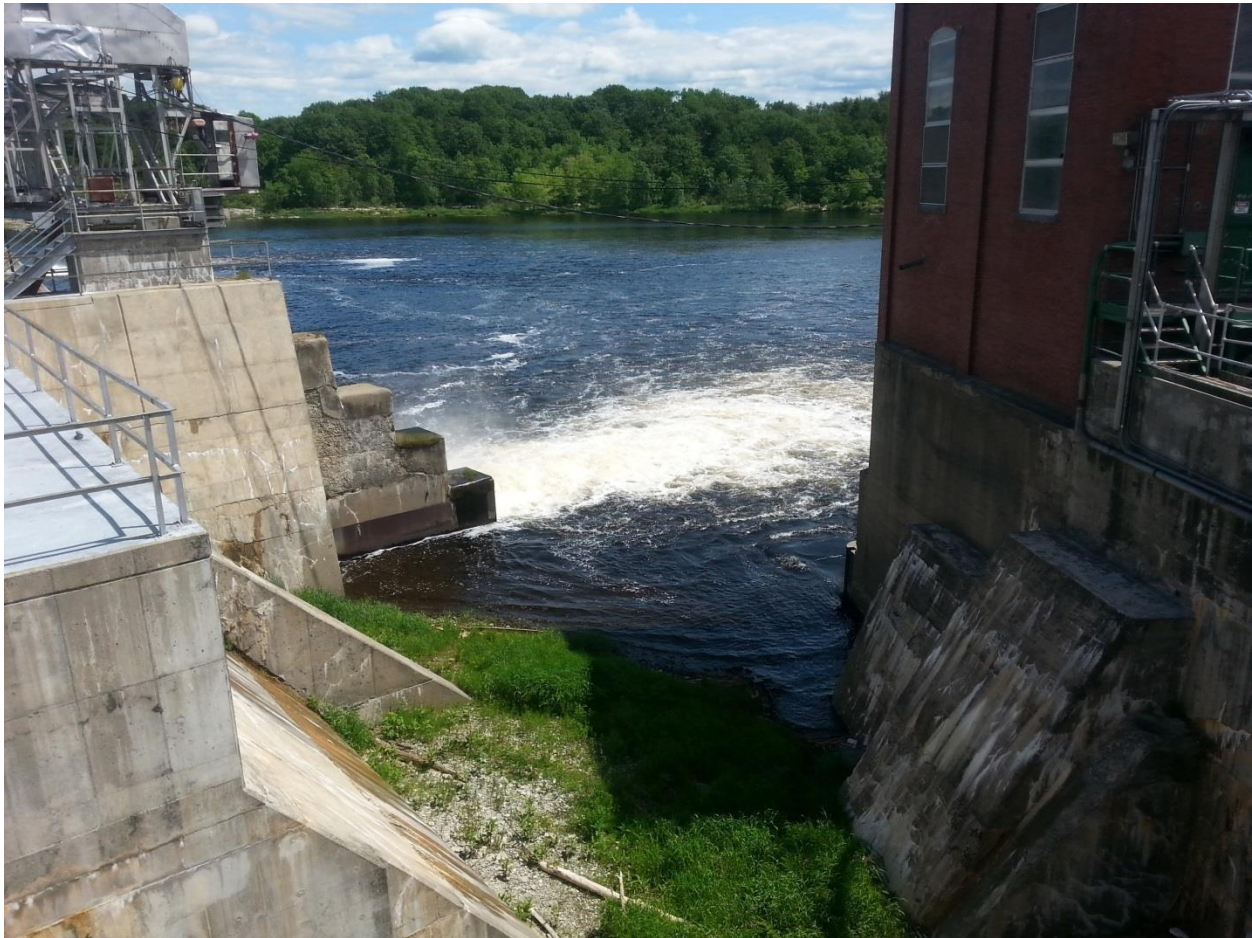
FIGURE 6: VIEW FROM WHERE THE NON-OVERFLOW DAM SECTION MEETS THE HEAD GATE STRUCTURE LOOKING TOWARD THE DOWNSTREAM SIDE OF THE NON-OVERFLOW PORTION OF THE DAM.
