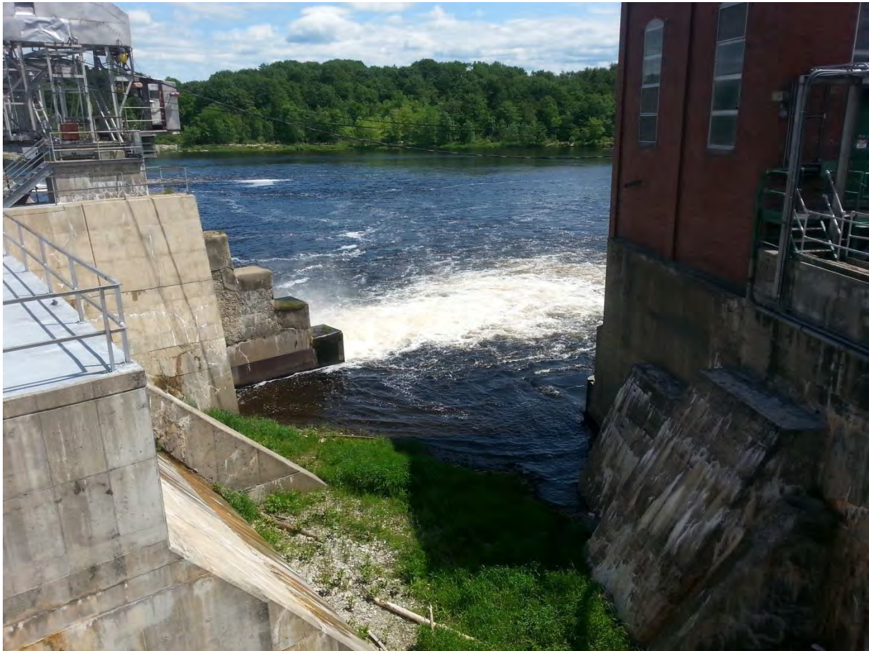
FIGURE 6: VIEW FROM WHERE THE NON-OVERFLOW DAM SECTION MEETS THE HEAD GATE STRUCTURE LOOKING TOWARD THE DOWNSTREAM SIDE OF THE NON-OVERFLOW PORTION OF THE DAM.
