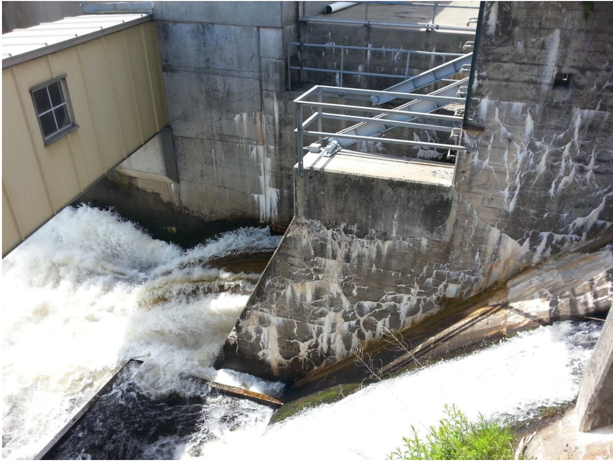
FIGURE 9: VIEW FROM AN ACCESS PLATFORM BEHIND THE UNITS 1 THROUGH 6 POWERHOUSE LOOKING AT THE DISCHARGE FROM THE TANTER GATE SHOWN IN FIGURE 8.
