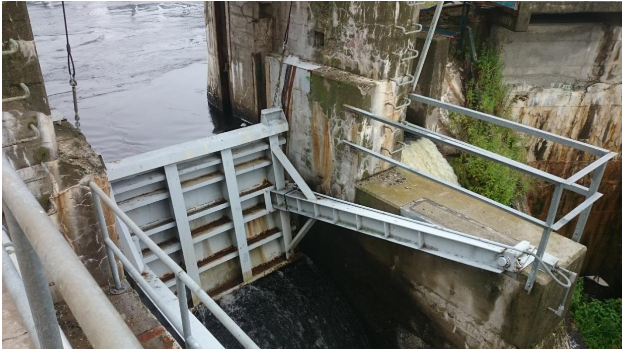
FIGURE 8: VIEW FROM AN ACCESS PLATFORM BEHIND THE UNITS 7 AND 8 POWERHOUSE LOOKING AT THE DOWNSTREAM FACE OF THE TAINTER GATE.
