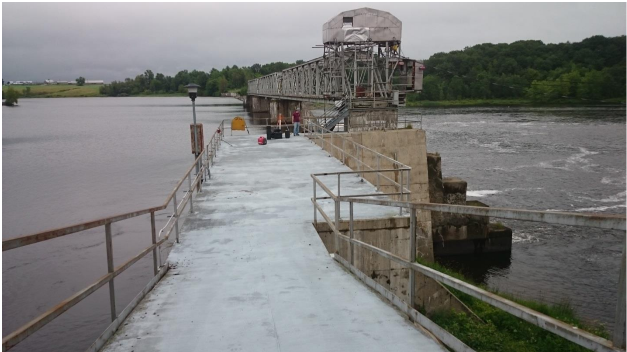
FIGURE 5: VIEW FROM THE TOP OF THE HEAD GATES LOOKING AT THE EXISTING CONCRETE DECK ABOVE THE NON-OVERFLOW PORTION OF THE DAM TO BE MODIFIED.
