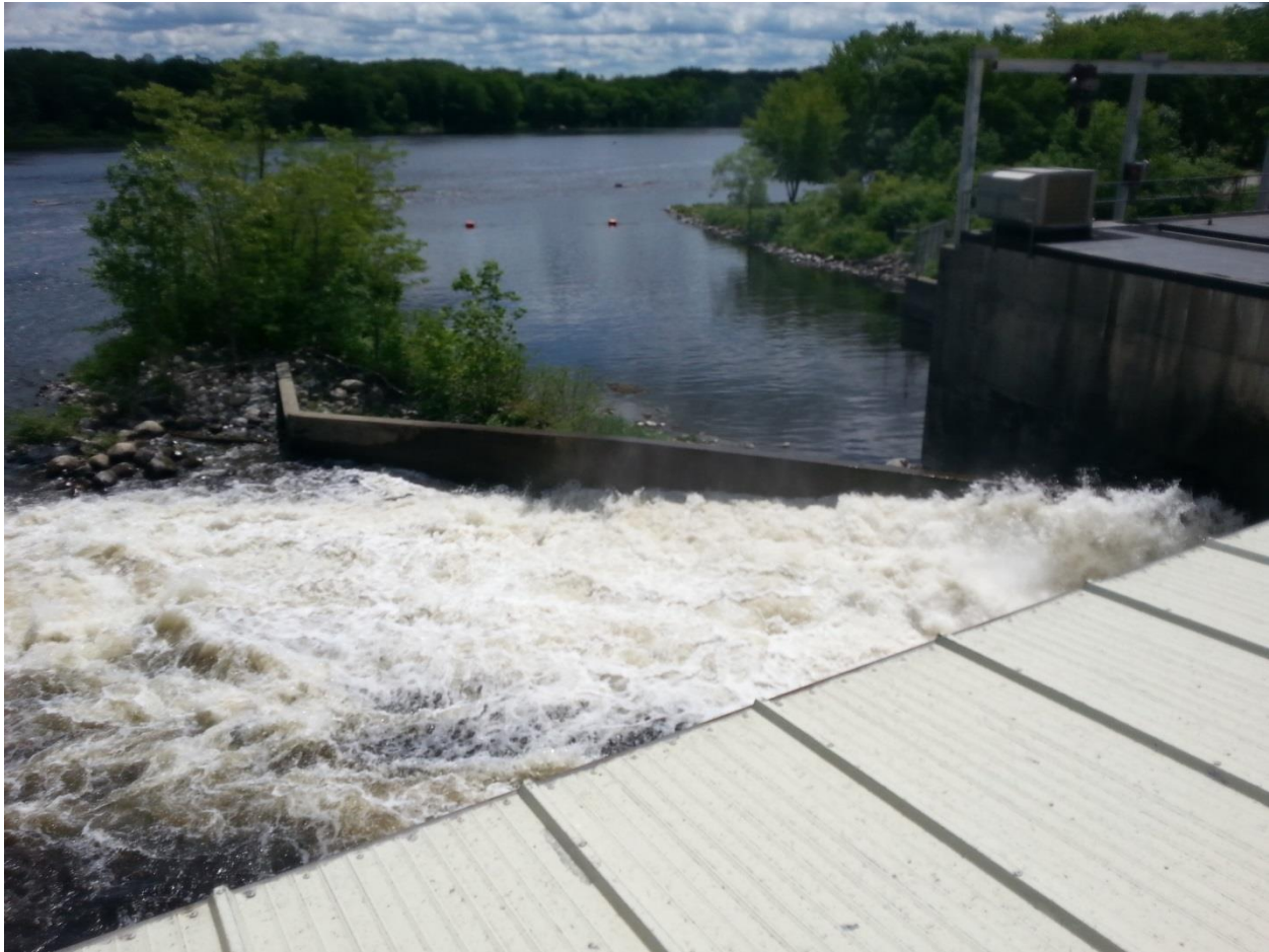
FIGURE 11: VIEW FROM THE PLATFORM ON THE DOWNSTREAM END OF THE FOREBAY BETWEEN THE TWO POWERHOUSES LOOKING DOWNSTREAM.
