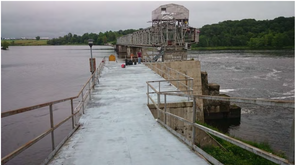
FIGURE 5: VIEW FROM THE TOP OF THE HEAD GATES LOOKING AT THE EXISTING CONCRETE DECK ABOVE THE NON-OVERFLOW PORTION OF THE DAM TO BE MODIFIED.
