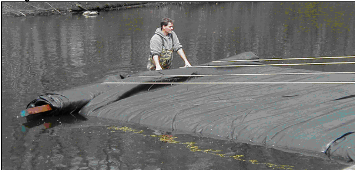
Figure 5.: A large AquaDam® being installed on the Saddle River in northeastern New Jersey. Only one laborer is needed in the water to keep the ropes in position. Using ropes require that the AquaDam® only be installed in a straight line. Connections can be made at a later date if turns are required. Coupling collars are placed underneath the first AquaDam® as it is being unrolled( if connections are necessary).
