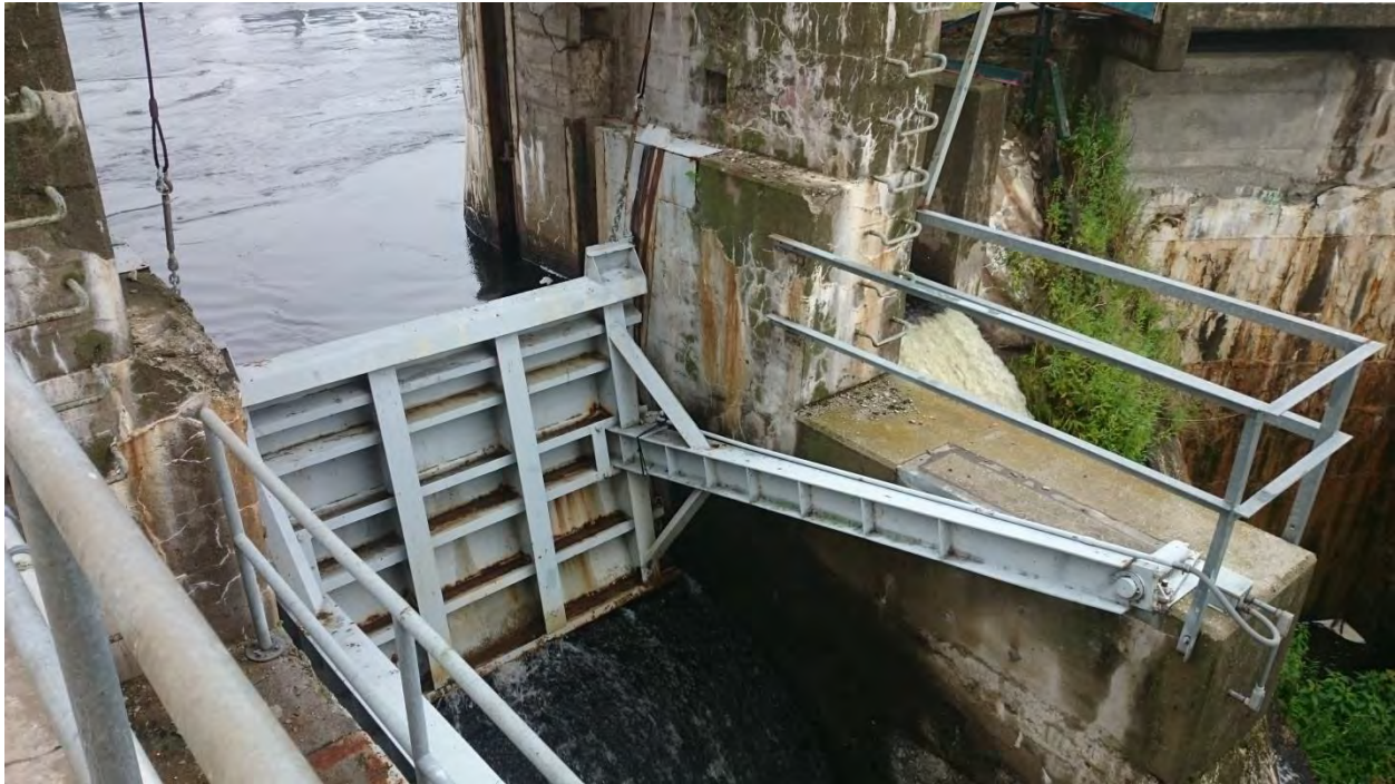
FIGURE 8: VIEW FROM AN ACCESS PLATFORM BEHIND THE UNITS 7 AND 8 POWERHOUSE LOOKING AT THE DOWNSTREAM FACE OF THE TAITER GATE.
