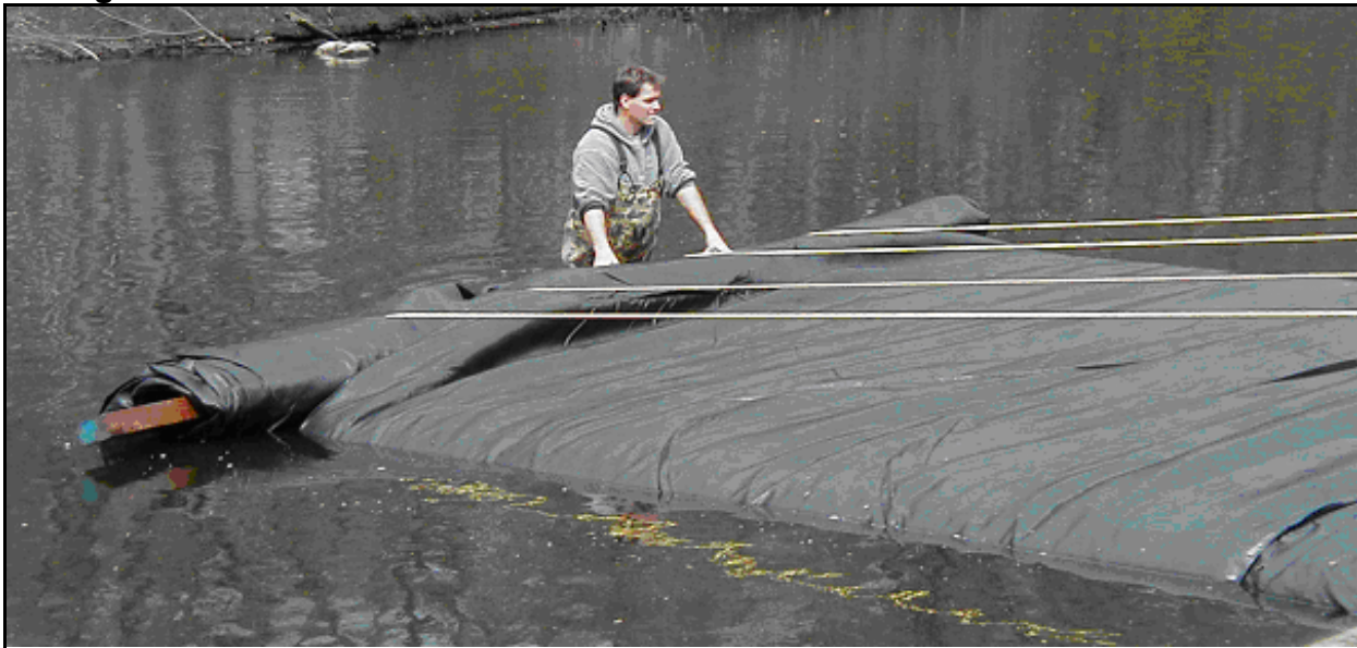
Figure 5.: A large AquaDam® being installed on the Saddle River in northeastern New Jersey. Only one laborer is needed in the water to keep the ropes in position. Using ropes require that the AquaDam® only be installed in a straight line. Connections can be made at a later date if turns are required. Coupling collars are placed underneath the first AquaDam® as it is being unrolled( if connections are necessary).
