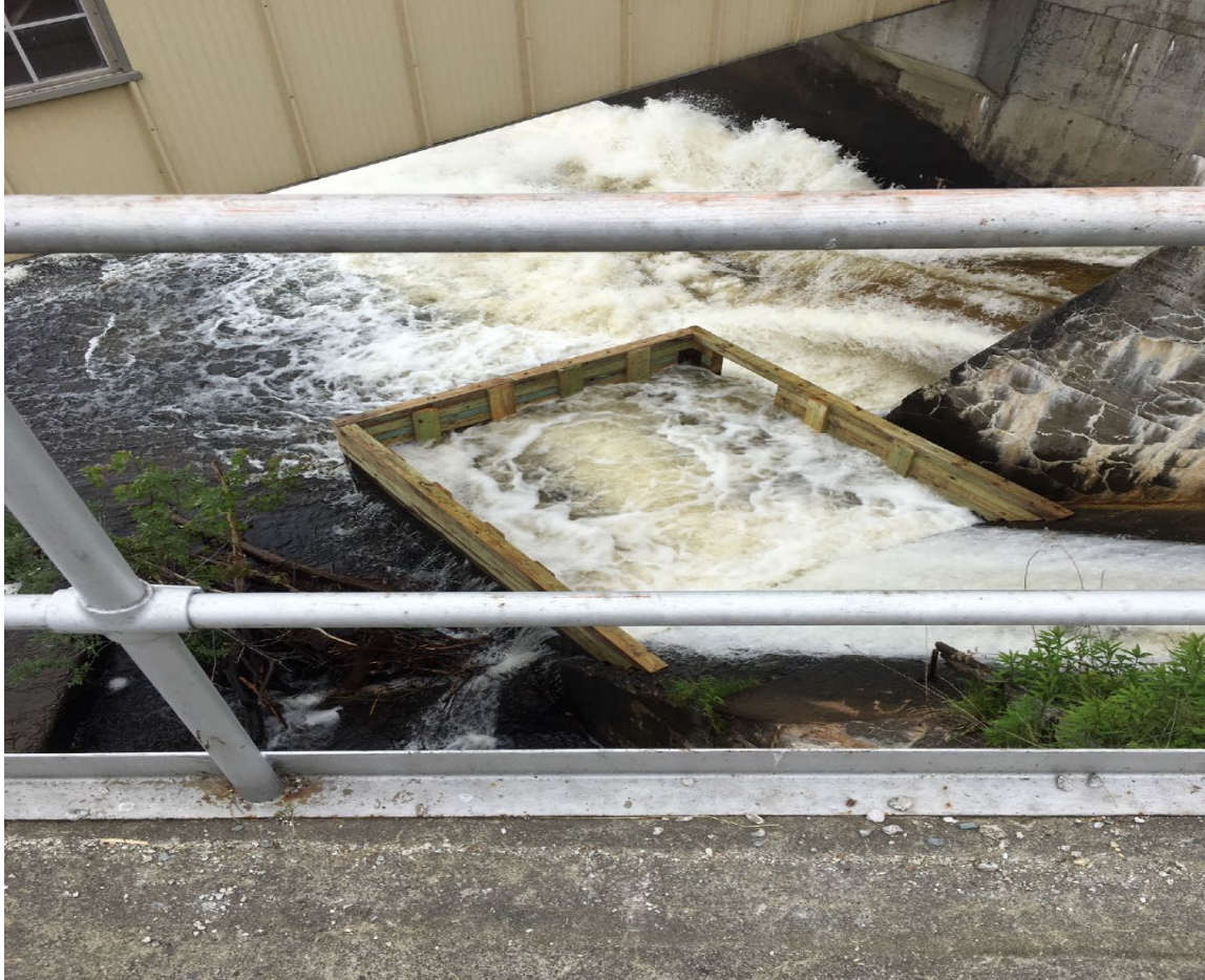
Figure 4. Plunge pool located immediately below the forebay bypass gates at the Shawmut Project. (Source: License Application).
