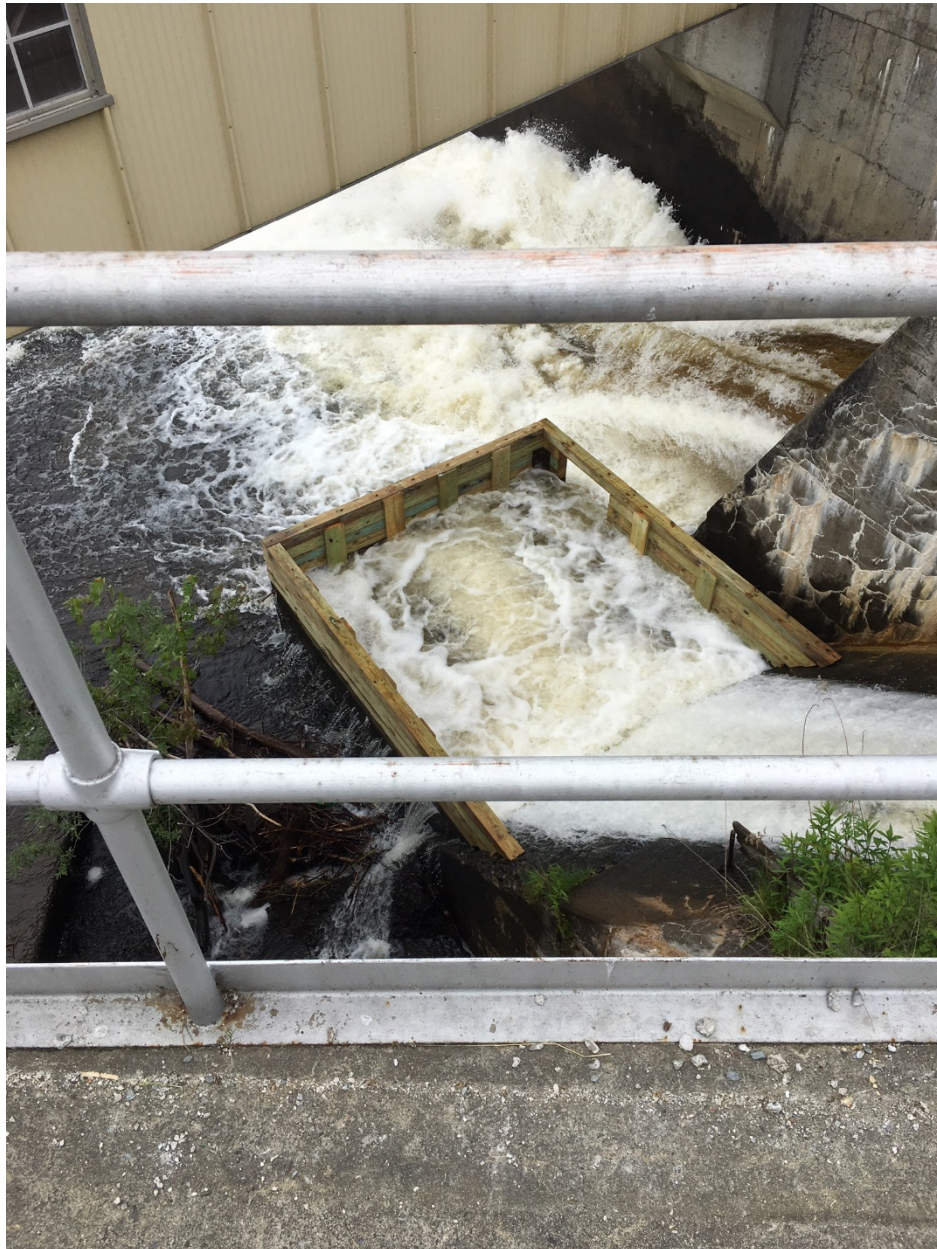
Photo 1. Shawmut Project Sluice Gate (near, boxed) and Tainter Gate (far) Plunge Pools.
