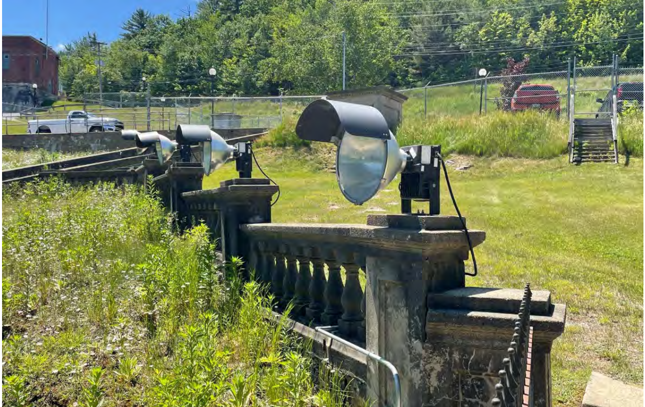
Figure 76: Lighting for falls at West Viewing Area.
