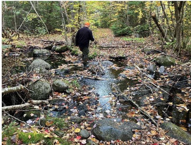
Figure 10. Example of needed access road repairs at a stream crossing adjacent to the West Branch below Stone Dam (October 10, 2024)
