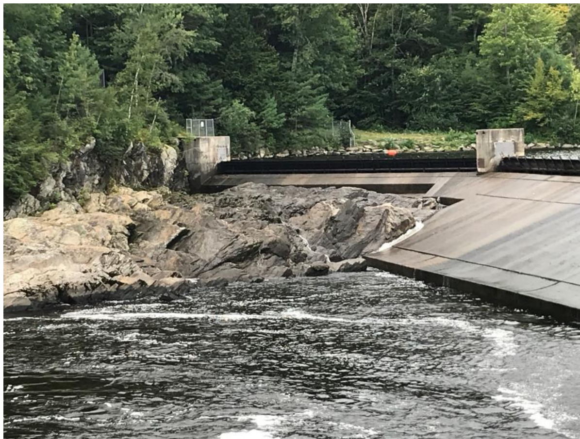
Figure 5.0-3: Exposed Bedrock Area Below Bascule Gate No. 5 (9:54 am)
