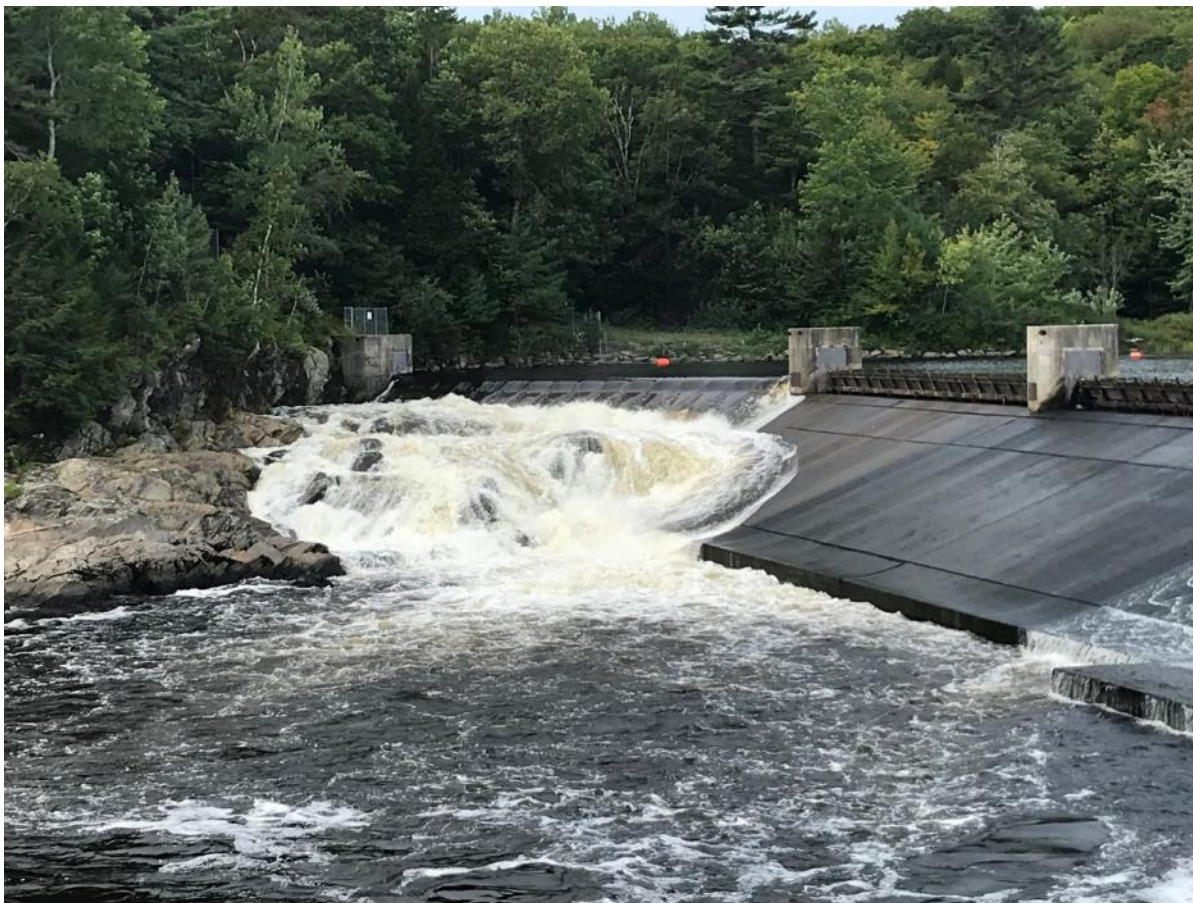
Figure 5.0-2: Bascule Gate No. 5 in Fully Lowered Position (9:37 am)
