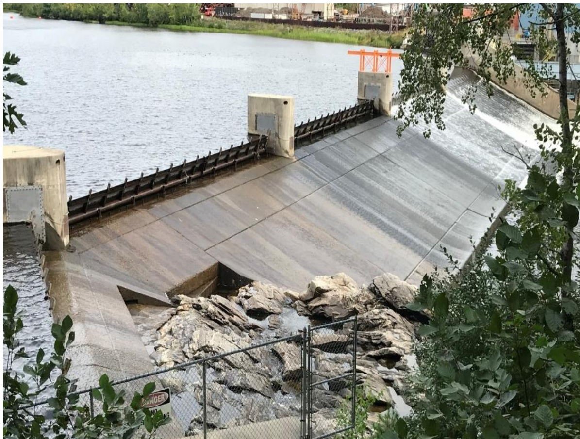
Figure 5.0-4: Exposed Bedrock Area Below Bascule Gate No. 5 (10:31 am)
