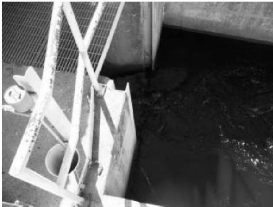
FIGURE 4 VIEW OF COLLECTION CHAMBER AND ENTRANCE TO DOWNSTREAM FISH PASSAGE PIPE AT THE ELLSWORTH DAM
