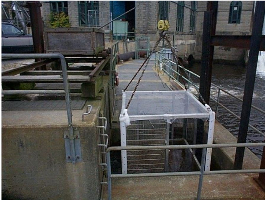
FIGURE 3 VIEW OF FISHWAY LIFT IN OPERATION USED FOR TRANSFERRING FISH TO THE HOLDING TANK AT THE ELLSWORTH DAM
