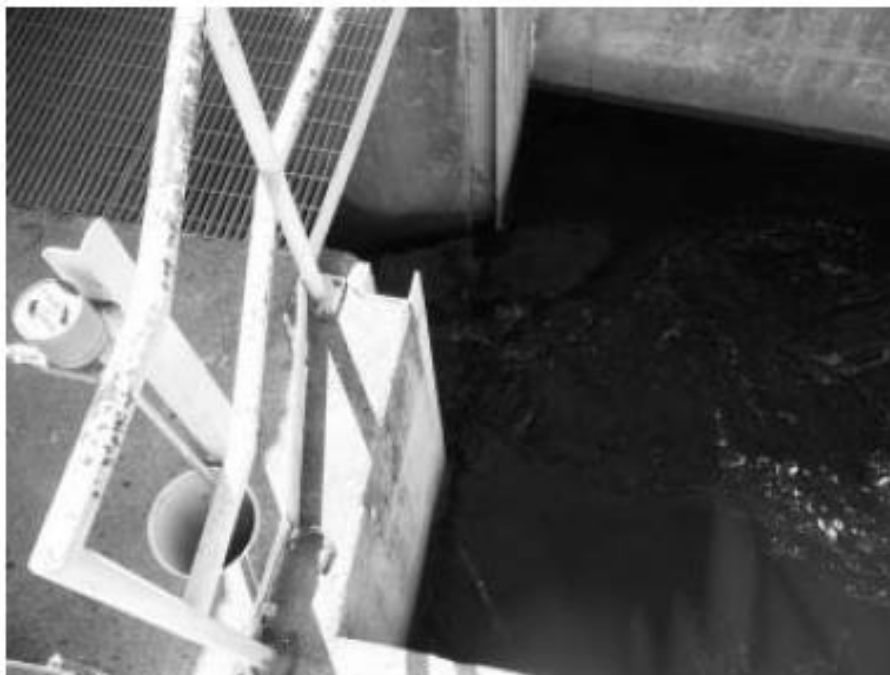
FIGURE 4 VIEW OF COLLECTION CHAMBER AND ENTRANCE TO DOWNSTREAM FISH PASSAGE PIPE AT THE ELLSWORTH DAM
