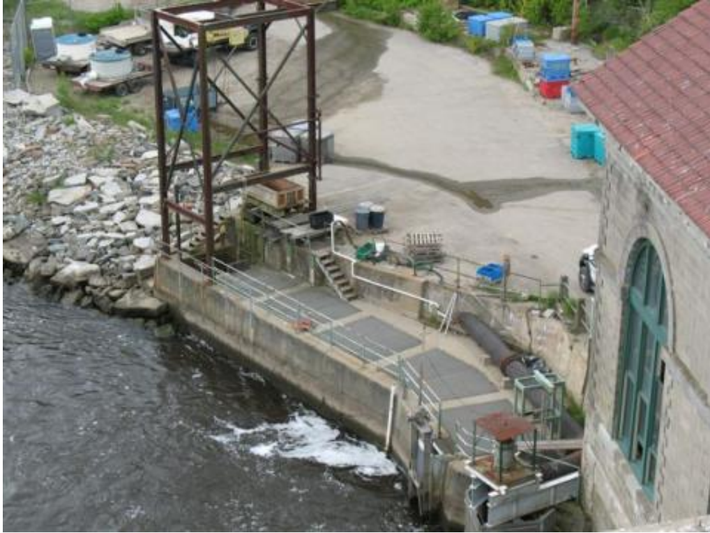
FIGURE 7 OVERVIEW OF FISHWAY TRAP AND TRANSFER FACILITY AT THE ELLSWORTH POWERHOUSE TAILRACE
