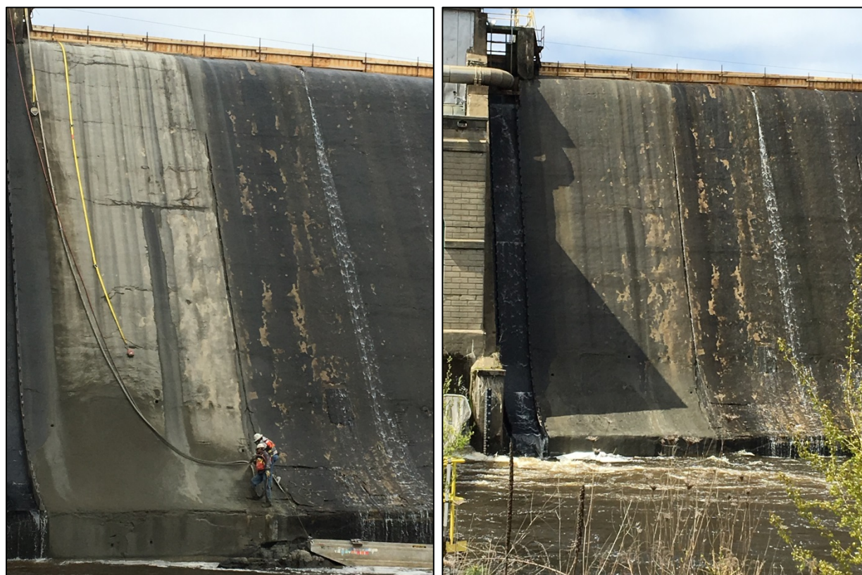
Figure 1-3. Ellsworth spillway face showing condition prior to study (top), concrete repair work (lower left), and final surface prior to opening of downstream bypass and additional flashboard spill during the 2017 study (lower right).
