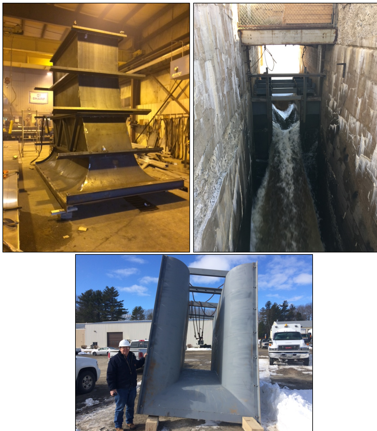
Figure 1-1. Alden weir installed into the downstream sluice at Graham Lake Dam. Photo on top left shows unit in build shop (oriented with the upstream entrance towards the shop floor and the weir floor facing the viewer), photo on top right shows the unit installed (as viewed from the downstream side of the sluice) and photo on bottom shows weir as viewed from upstream looking down through.
