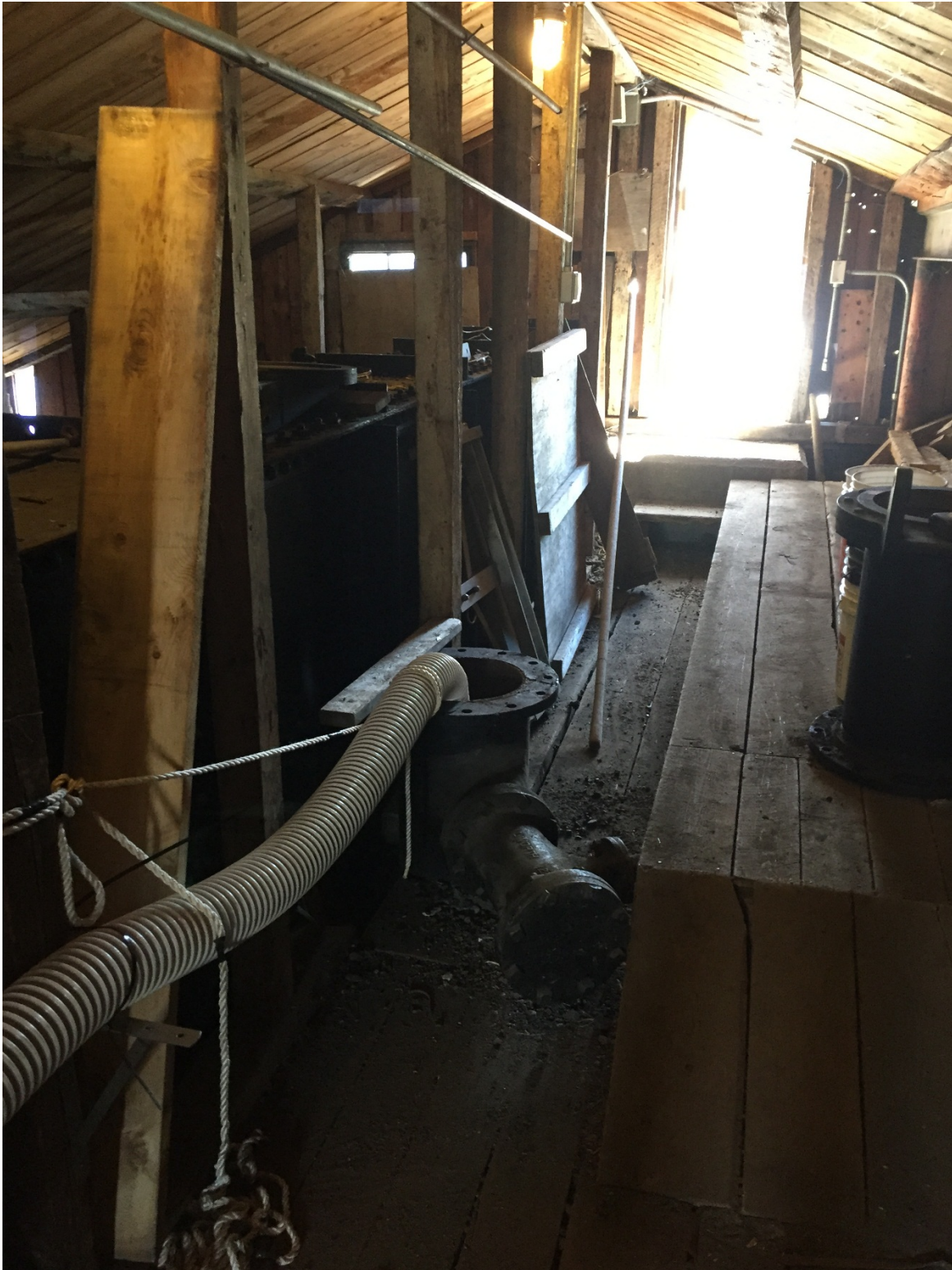
Figure 3.4. A 4-inch release hose was installed into a vent pipe into the penstock of turbine Unit 1. A similar release hose was lowered into a vent slot into the penstock of turbine Unit 2 and the downstream bypass.
