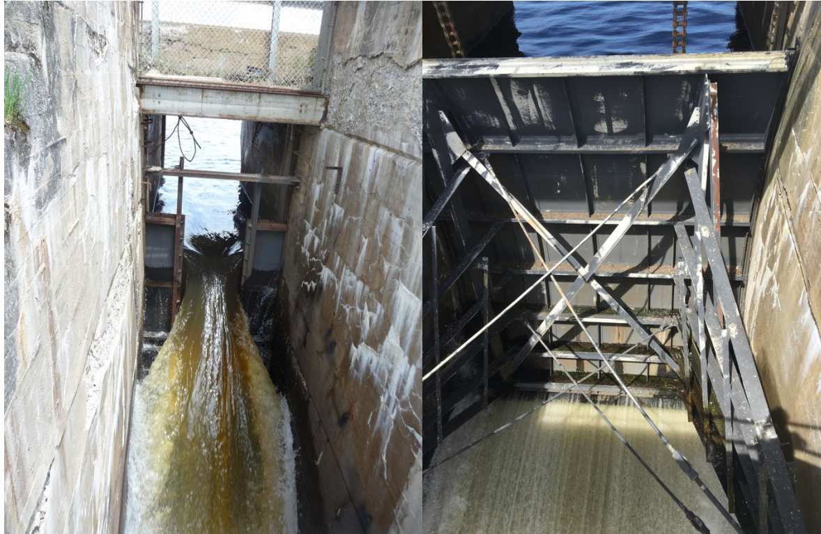
Figure 4-6. Downstream bypass sluice with stop logs removed and bottom opening radial gate at Graham Lake Dam during the study period May 11-May 31, 2016.
