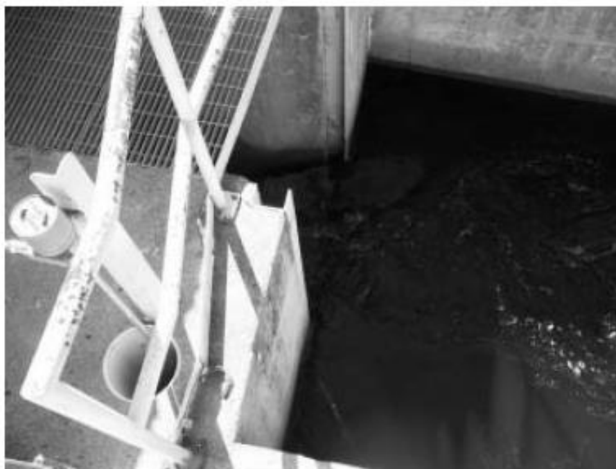
FIGURE 4 VIEW OF COLLECTION CHAMBER AND ENTRANCE TO DOWNSTREAM FISH PASSAGE PIPE AT THE ELLSWORTH DAM
