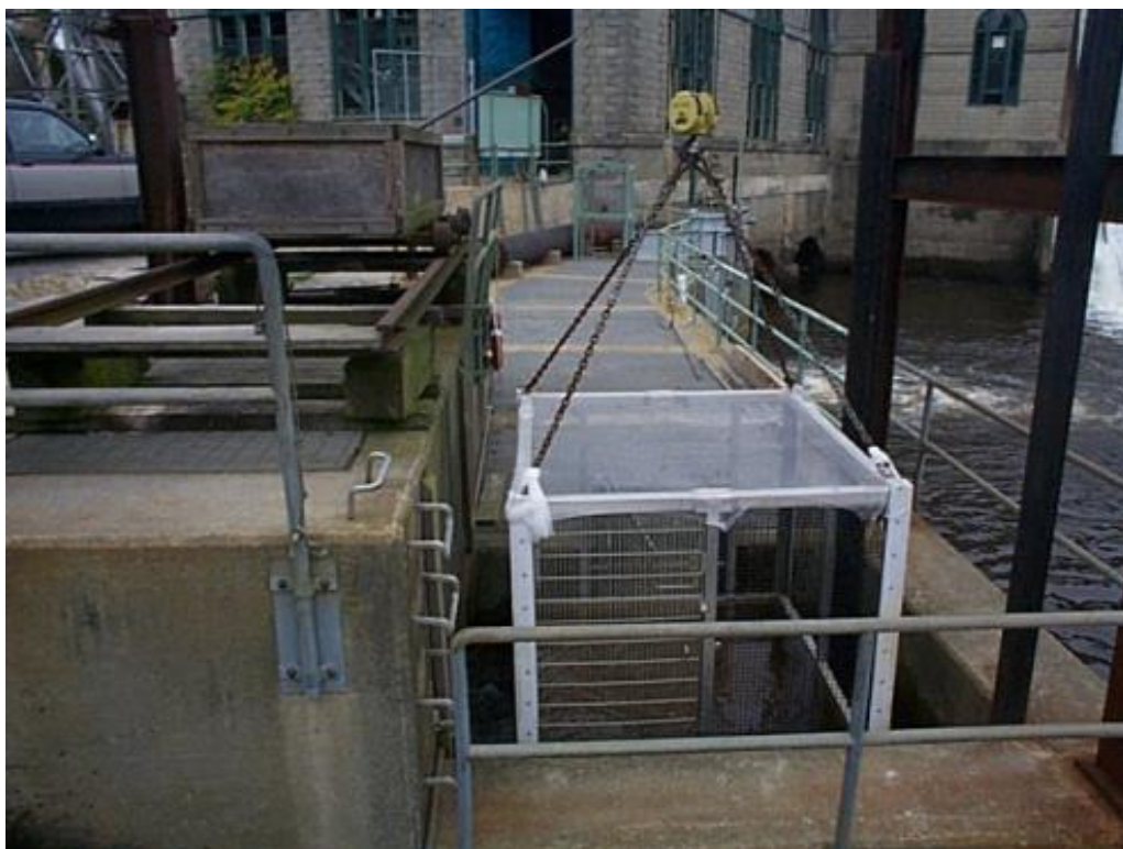
FIGURE 6 VIEW OF FISHWAY HOPPER IN OPERATION USED FOR TRANSFERRING FISH TO THE HOLDING TANK AT THE ELLSWORTH DAM
