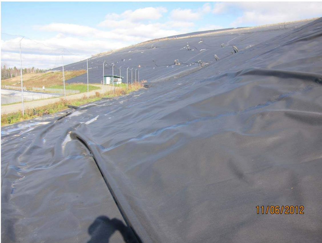
SW corner looking north along western slope of Cells 1&2 (Cell 4 in foreground)
