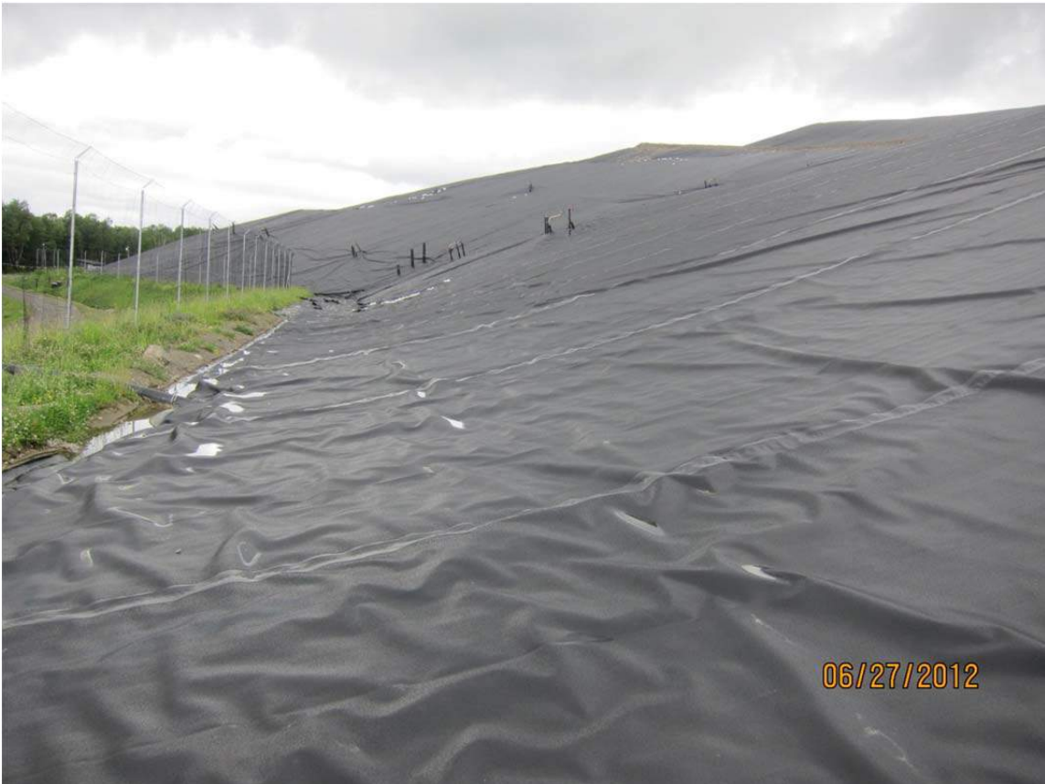
SW corner of Cell 4, looking northwest along lower southwestern slope of Cell 4
