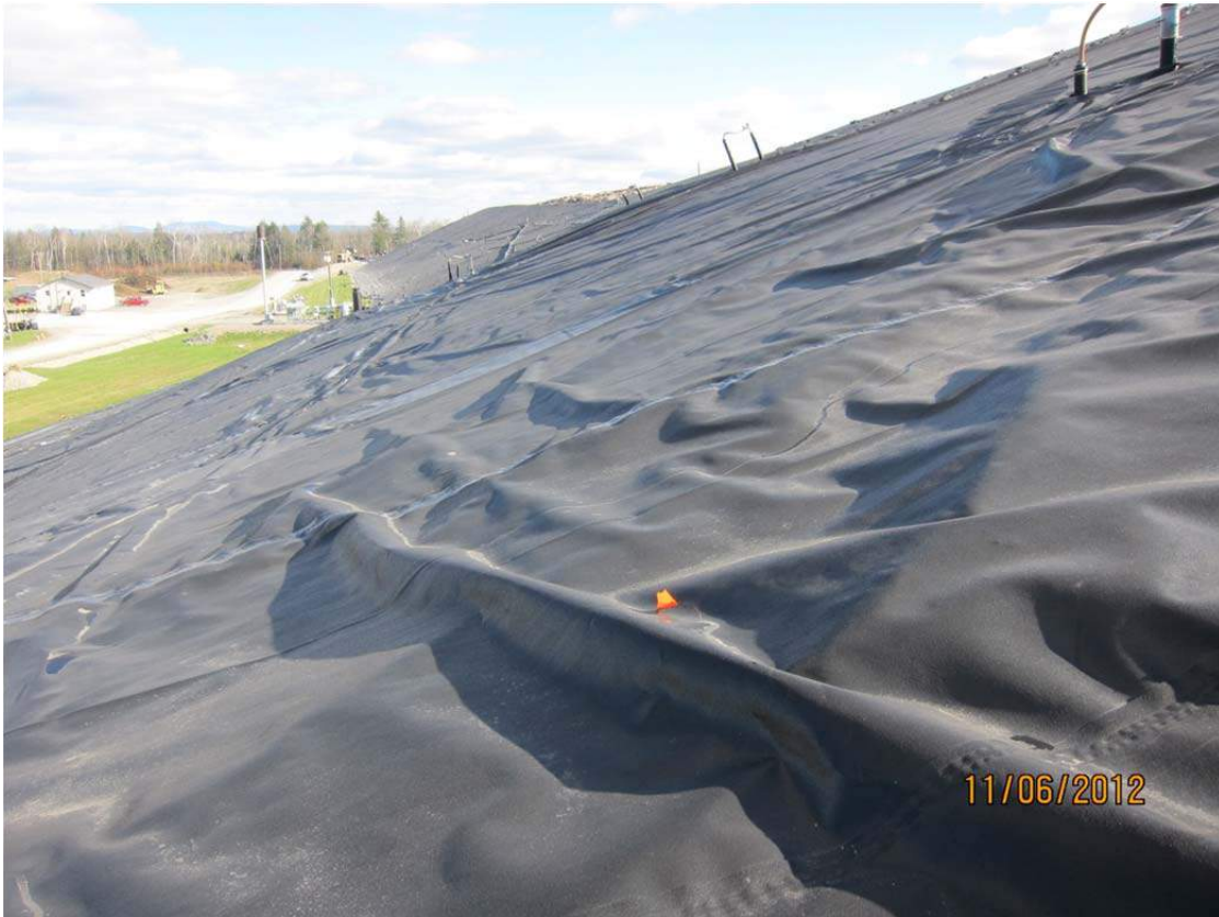
NW corner looking east along northern slope of Cell 1 & 2 (foreground) Cell 3 (background)
