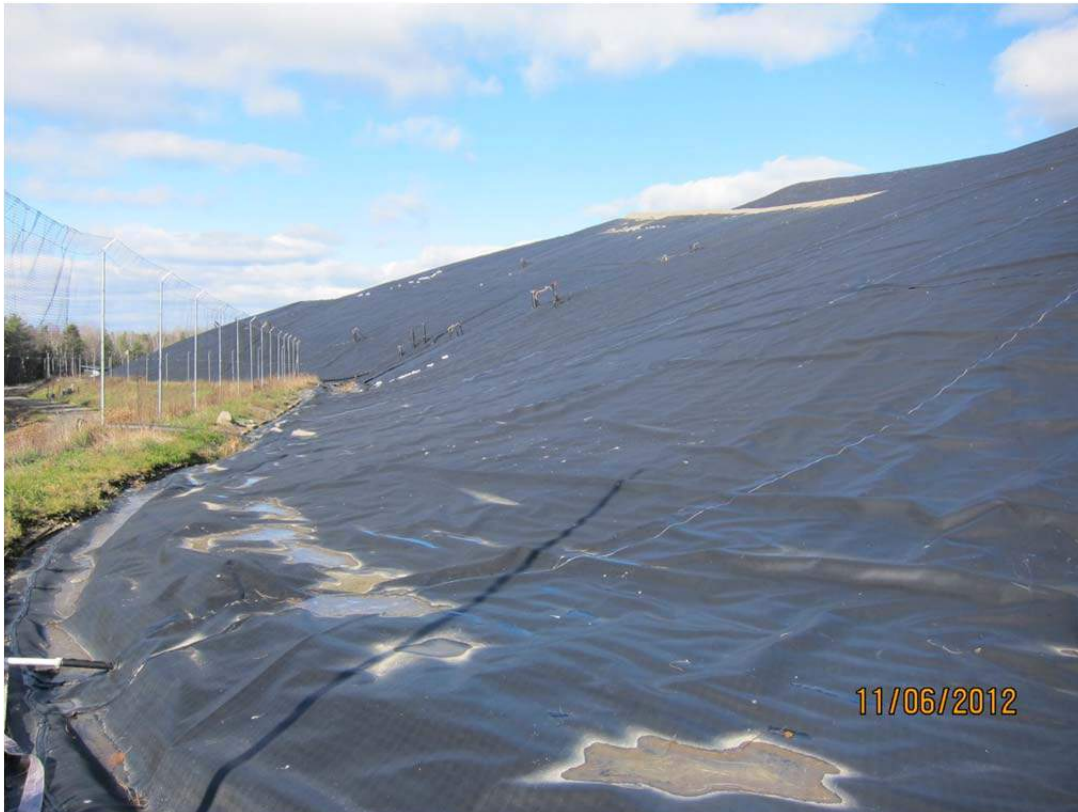
SW corner of Cell 4, looking northwest along lower southwestern slope of Cell 4
