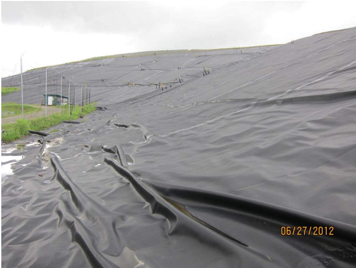
SW corner looking north along western slope of Cells 1&2 (Cell 4 in foreground)
