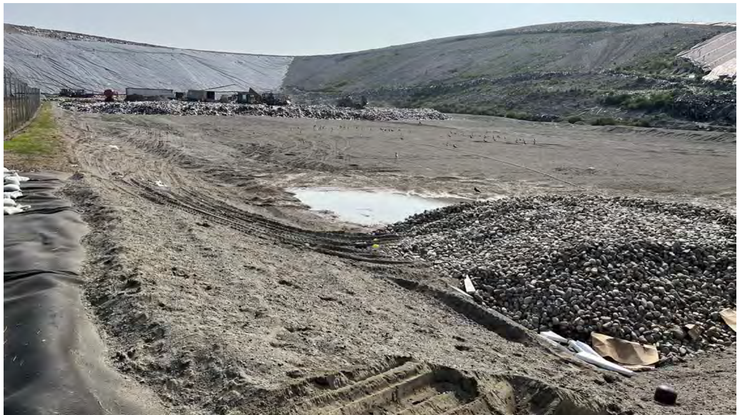
46. at the southwest corner of Cell 15, looking at Cell 15 foundation and the slopes of Cells 1/2/3/7/12/13/14
