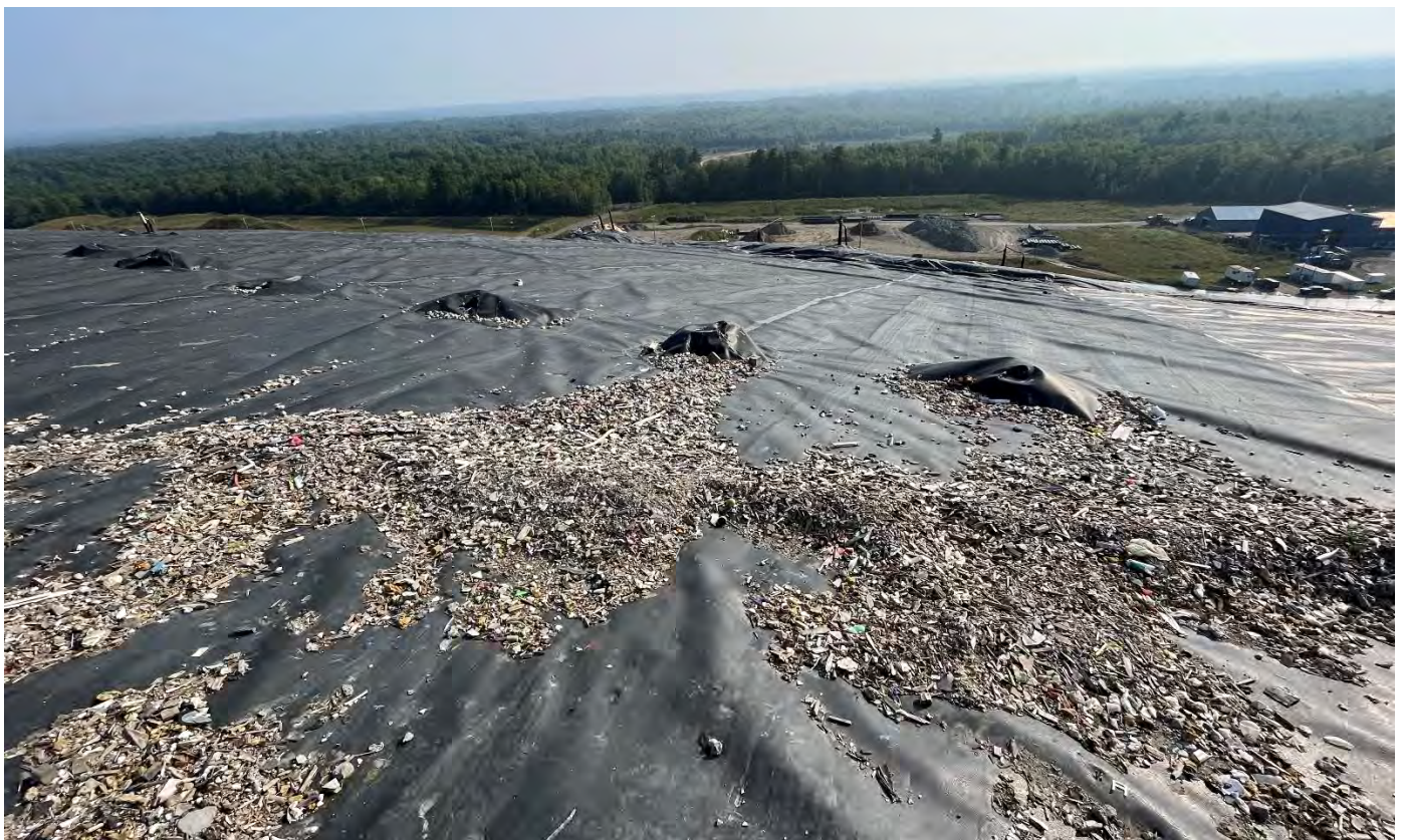
6. top of the south end of Cell 10 looking easterly down northeasterly slope of Cell 10
