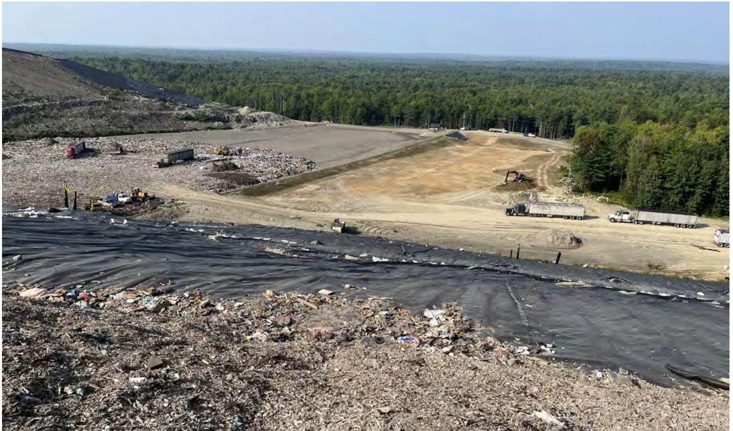
21. on the southwesterly slope of Cell 13/14 looking south towards the next area of Cell 16 construction
