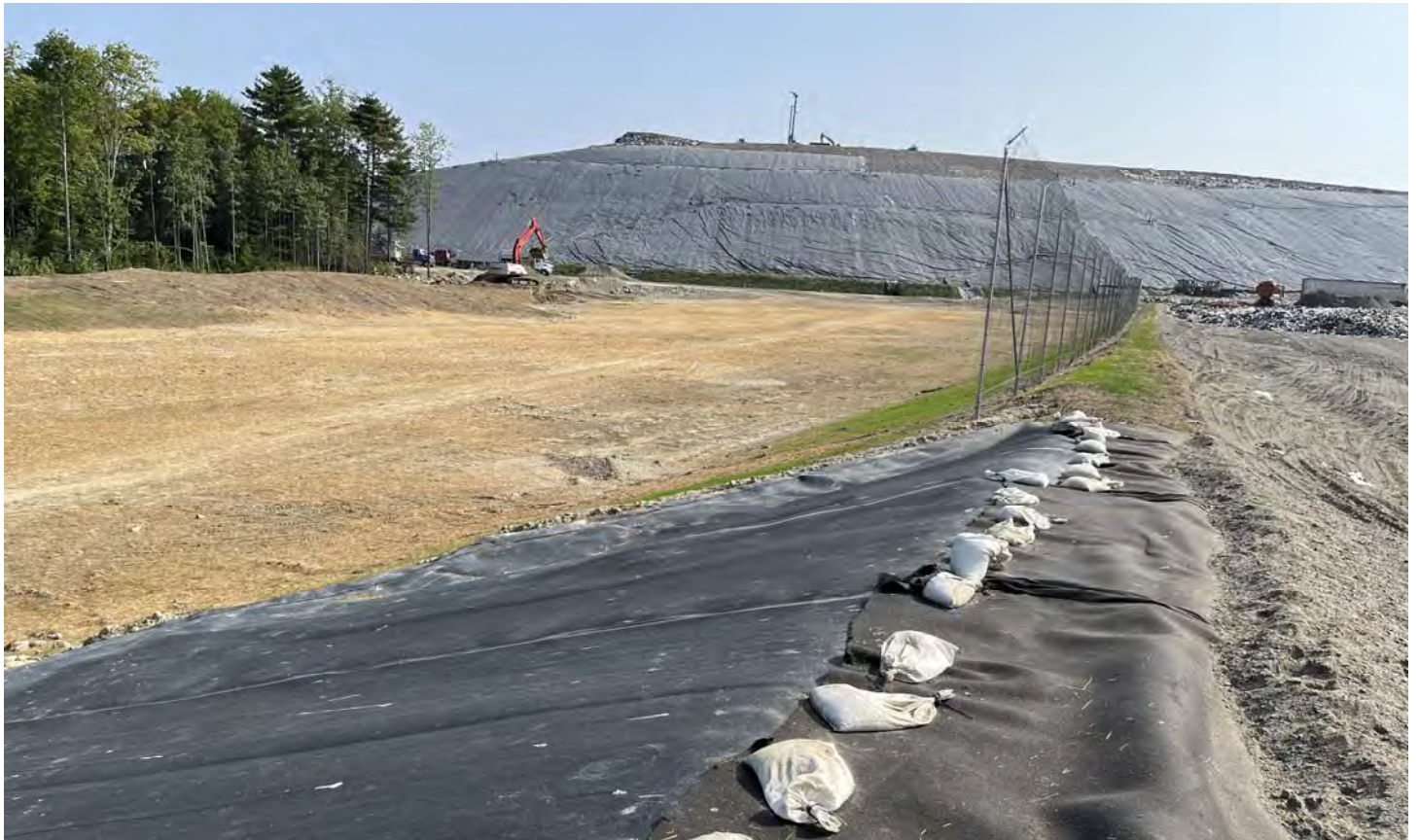
47. looking along the east/west boundary of Cell 15 and the southwesterly slopes of Cells 12/13/14
