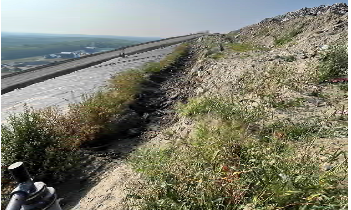
9. mid-height of Cell 11 looking southerly along upper easterly slope of Cell 11
