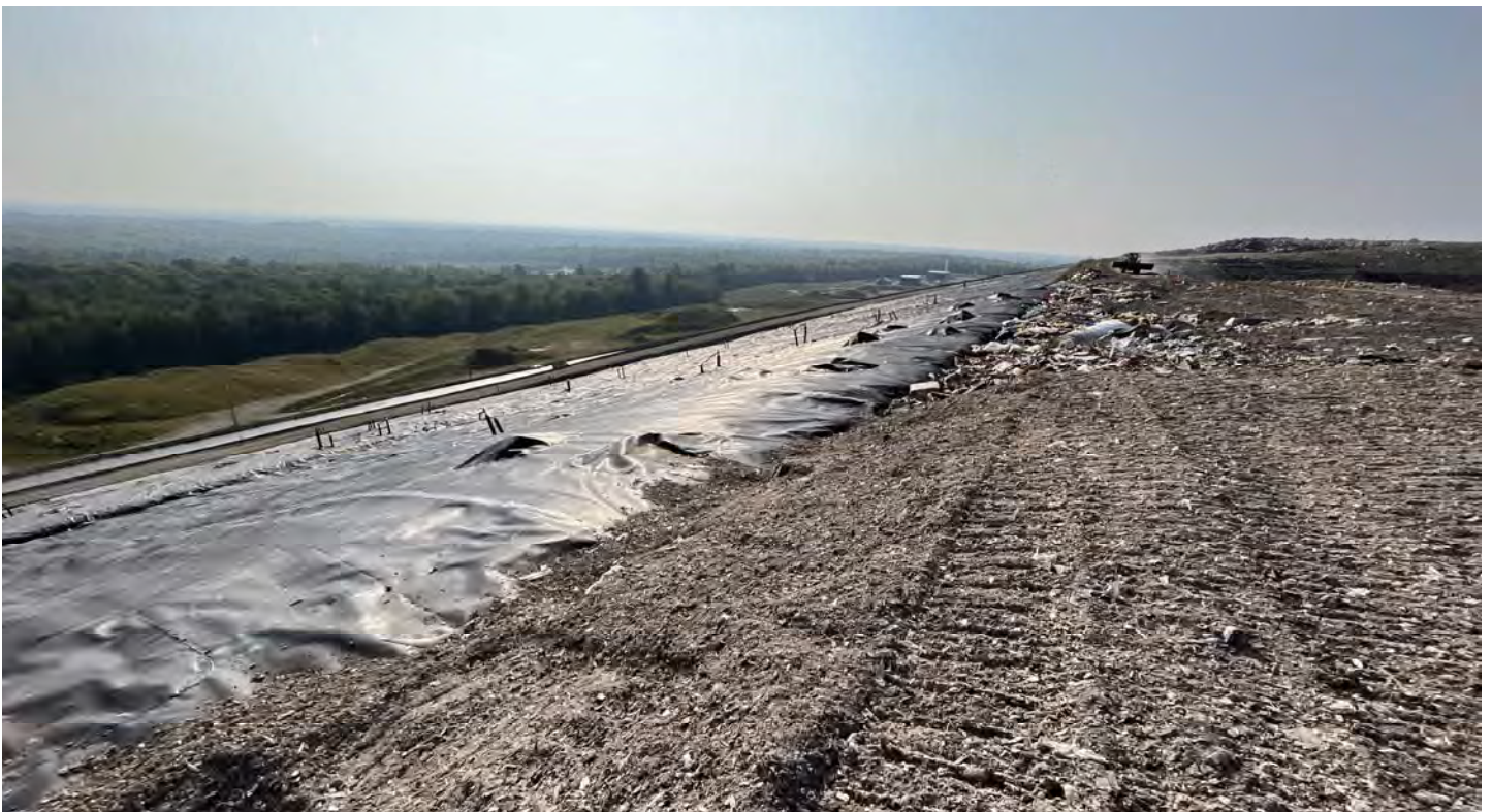
10. top of Cell 12 looking southeasterly along the easterly upper slope of Cells 12/11
