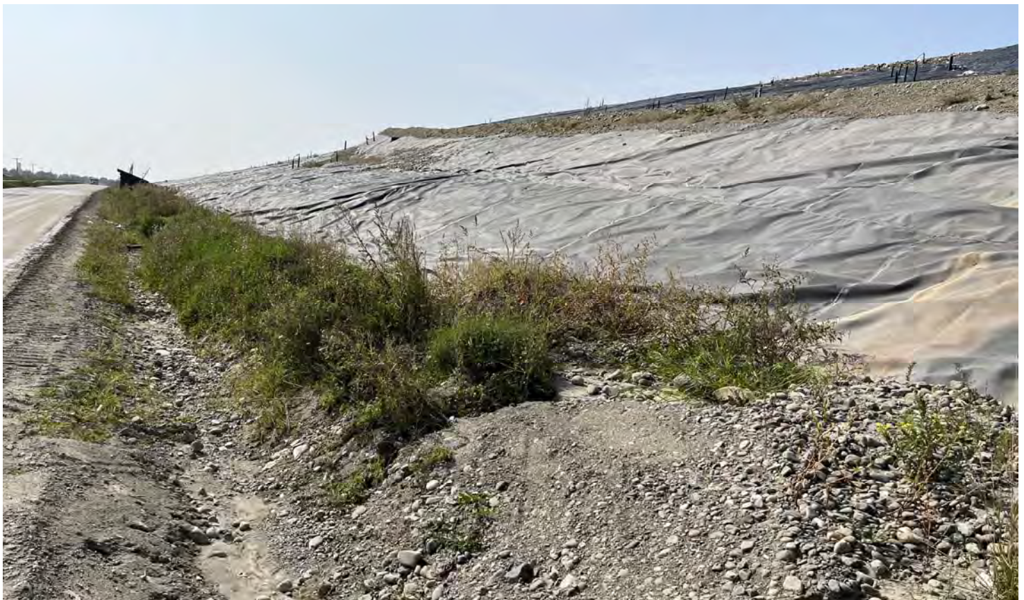
52. along the southeast access road, looking southeasterly along the eastern slopes of Cells 13/12/11
