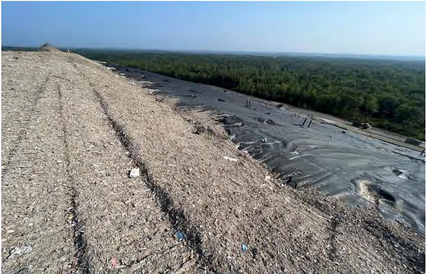
11. top of Cell 12 looking northeasterly along the easterly upper slope of Cells 12/13/14
