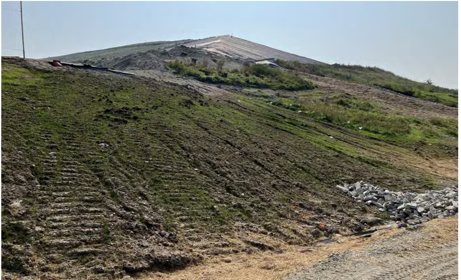
43. at the northwest landfill corner, looking easterly up the east/west ridge line of Cells 1/2
