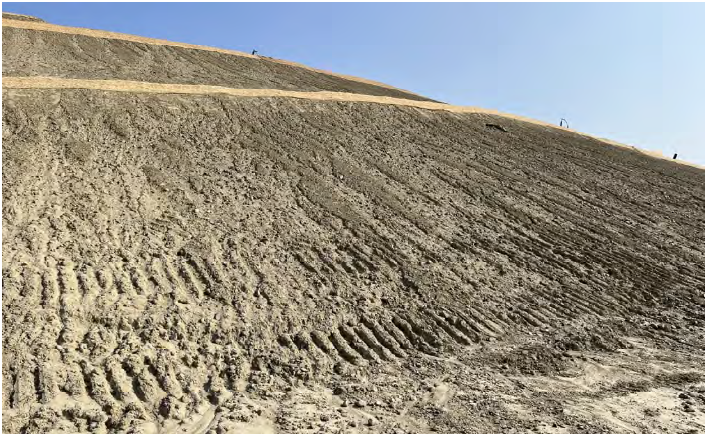
32. looking upwards towards the closure grading of the southerly facing slope at toe of Cell 10
