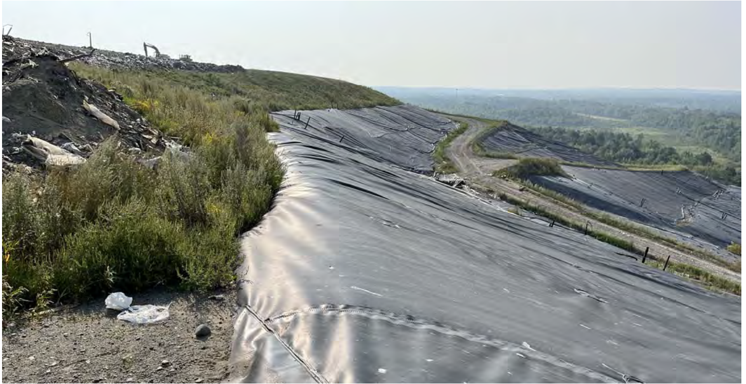
25. mid-height of southwest ridge line, looking southeasterly along the mid to upper slope of Cells 1/2/3A
