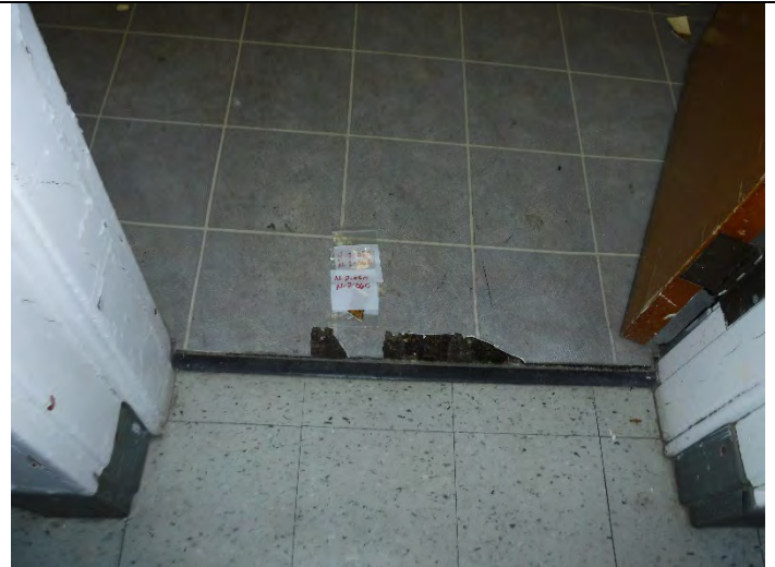
Photo 12 (12-16-2021): ACM mastic (NO-2-06) associated with PACM linoleum (NO-2-05) in North Wing – Section II.
