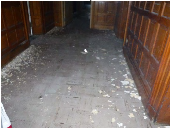
Photo 3 (12-15-2021): Administrative building/area. 9-inch VFT mottled tan. Floor tiles positive, ACM sample AD-2-01; associated mastic negative (AD-2-02).
