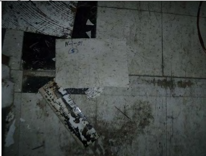
Photo 1 (12-16-2021): ACM 9-inch floor tile (NO-1-01) and associated ACM mastic (NO-1-02) located in select room of North Wing – Section I
