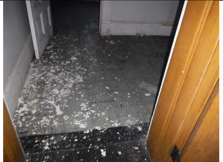
Photo 2 (12-15-2021): Administrative building/area. 9-inch VFT brown with black mottles. Floor tiles positive, ACM sample AD-1-03; associated mastic negative (AD-1-04).
