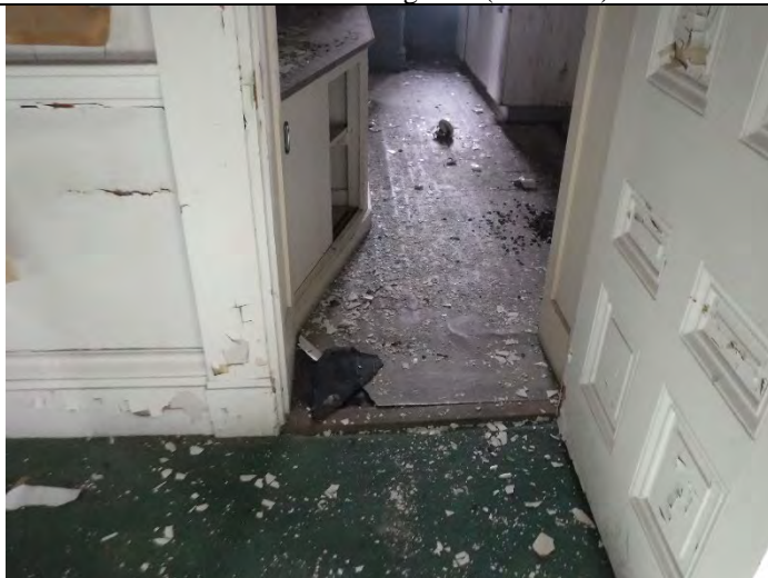
Photo 5 (12-15-2021): Administrative building/area. Kitchen linoleum. Associated mastic positive, ACM sample AD-3-10; impacted linoleum PACM (AD-3-09).
