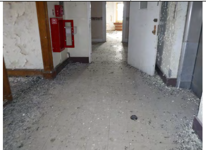
Photo 6 (12-15-2021): Administrative building/area. 9-inch VFT tan. Floor tile positive, ACM sample AD-4-01; associated mastic negative (AD-4-02).
