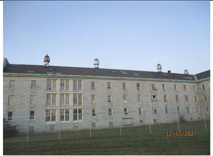
Photo 2 (12-17-2021): South Wing – Section I. South Wing – Section II on far right and out of photo.
