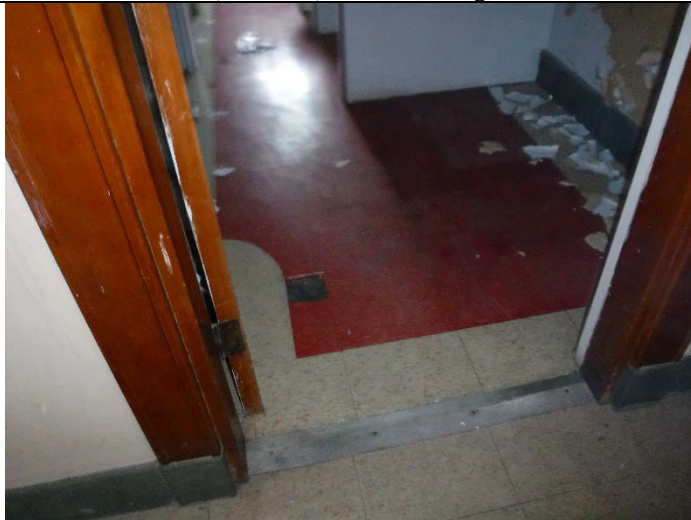
Photo 11 (12-16-2021): ACM black mastic (NO-2-03-Layer 2) associated with PACM 12-inch floor tile in North Wing – Section II.
