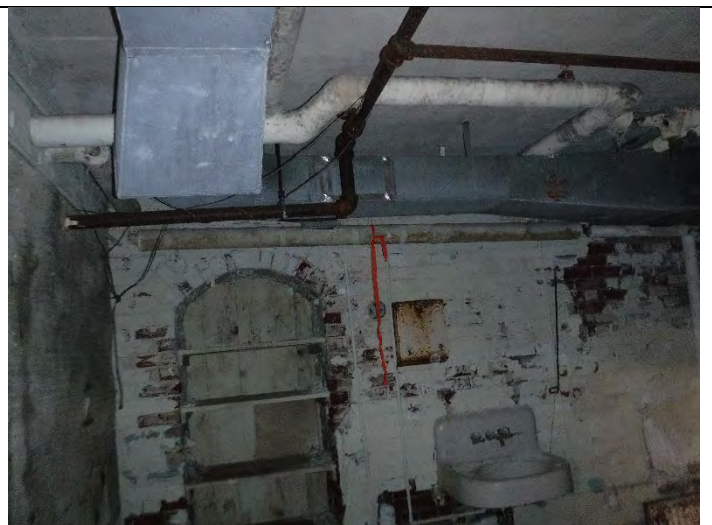
Photo 4 (12-17-2021): One of several areas of flagged ACM TSI within rooms off main corridors in basement area.
