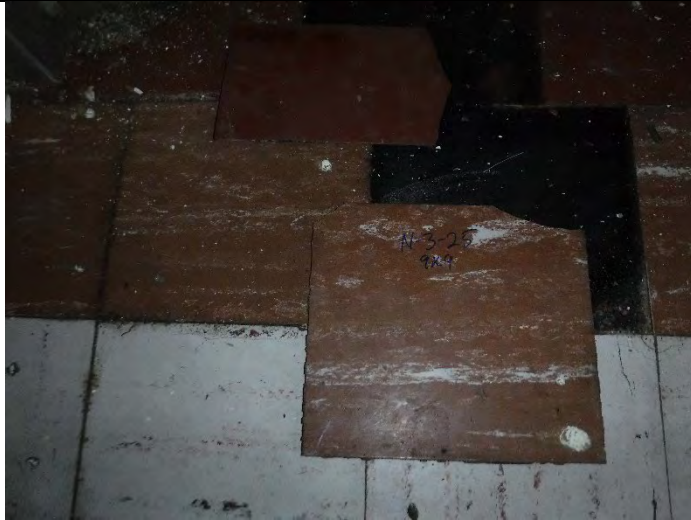
Photo 7 (12-16-2021): Three types of ACM or PACM 9-inch floor tile (NO-3-24, NO-3-25), all associated with ACM mastics located in North Wing – Section III.
