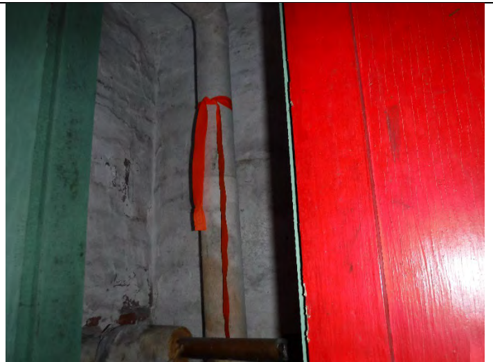
Photo 6 (12-17-2021): One of several areas of flagged ACM TSI within rooms off main corridors in basement area.
