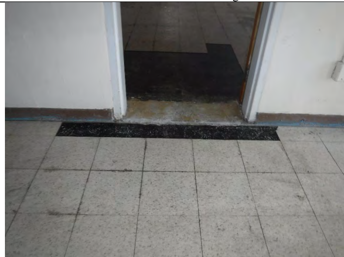
Photo 3 (12-17-2021): ACM 9-inch floor tiles (SO-2-01) and associated ACM mastic (SO-2-02) discovered beneath an area of 12-inch floor tiles (NAD). South Wing – Section III.
