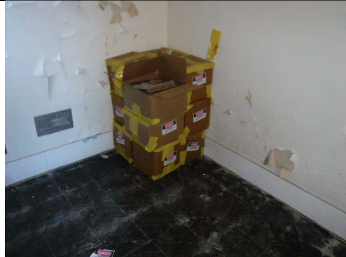
Photo 1 (12-17-2021): Boxed and labeled ACM flooring, located on first floor of South Wing – Section I
