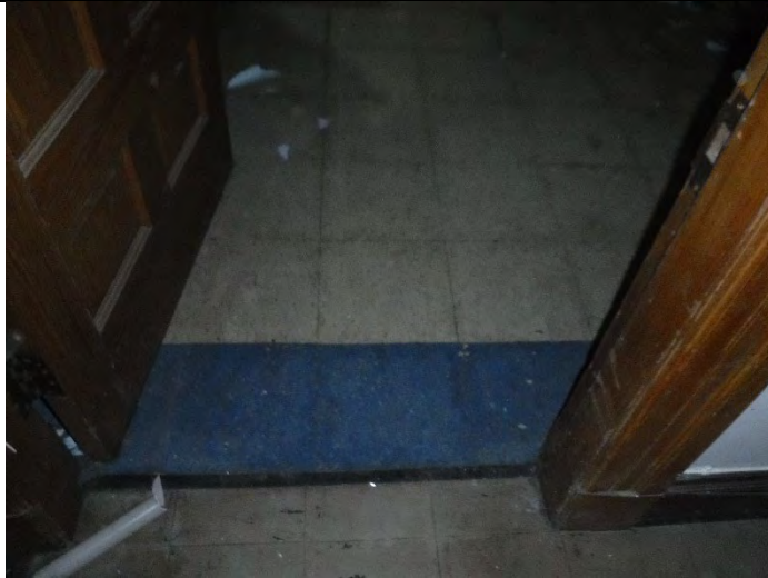
Photo 1 (12-15-2021): Administrative building/area. 9-inch VFT blue, mottled. Floor tile positive, ACM sample AD-1-01; associated mastic negative (AD-1-02).
