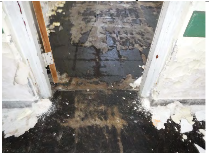
Photo 4 (12-17-2021): ACM thick black mastic (SO-3-02) located in select rooms/areas of South Wing – Section III.
