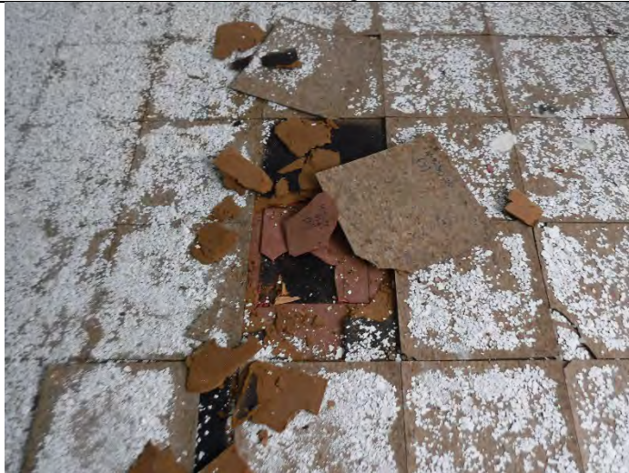
Photo 9 (12-16-2021): ACM 12-inch floor tile (NO-3-30) overlying ACM 9-inch floor tile (NO-3-31) and associated ACM mastic (NO-3-29) in North Wing – Section III.
