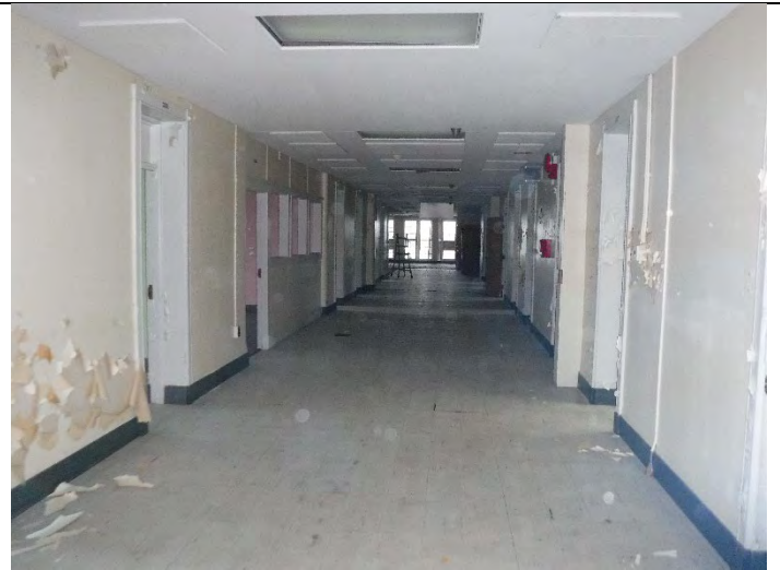
Photo 2 (12-16-2021): ACM 9-inch floor tile (NO-3-01) located throughout hall/rooms of North Wing – Section I.
