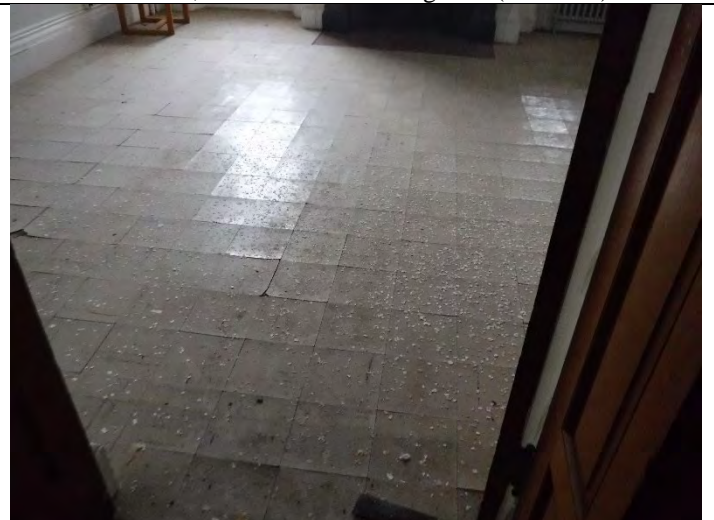
Photo 4 (12-15-2021): Administrative building/area. 9-inch VFT mottled gray. Associated mastic positive, ACM sample AD-2-04; floor tiles PACM (AD-2-03).
