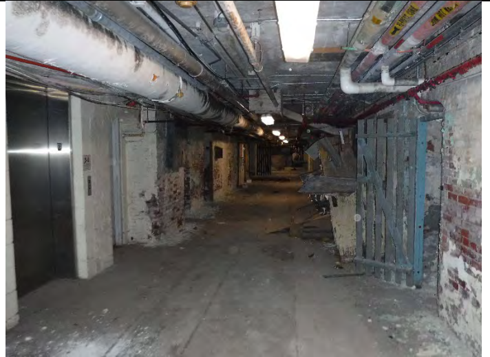
Photo 2 (12-17-2021): Basement corridors with labeled ACM TSI piping runs of various sizes.
