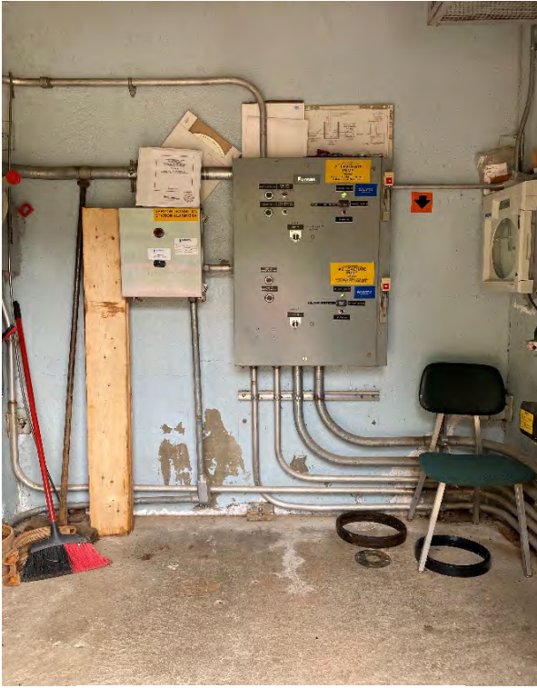
Leachate Pump Station Controls
