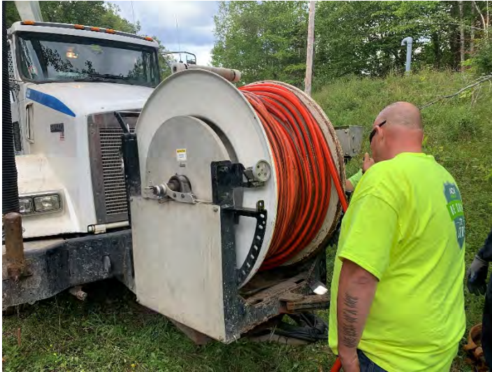
Dirty Line at Manhole 10
