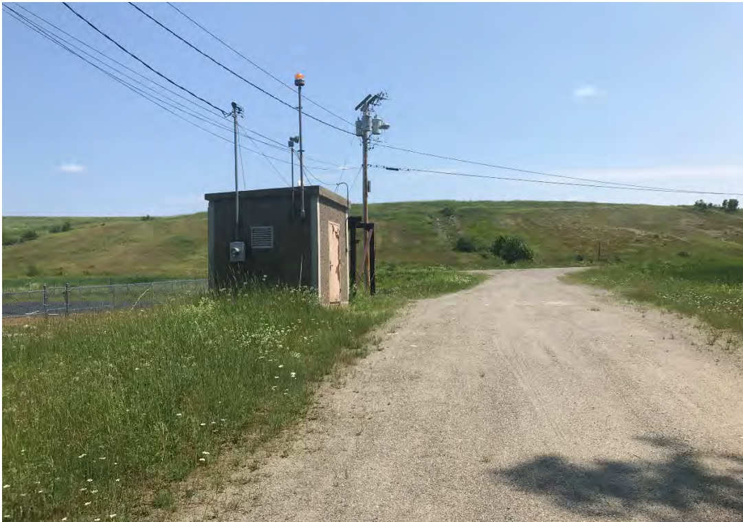
Leachate Pond Pump Station
