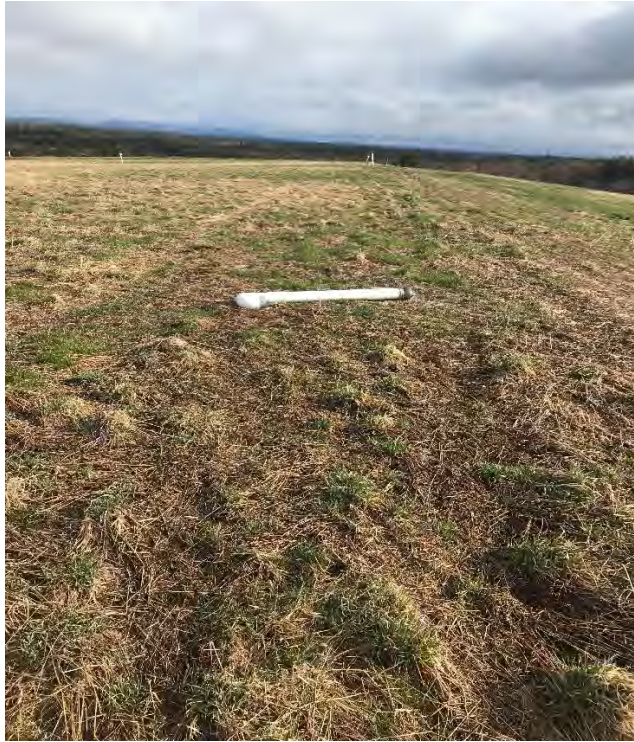
Dolby III Gas Vent (To Be Repaired)
