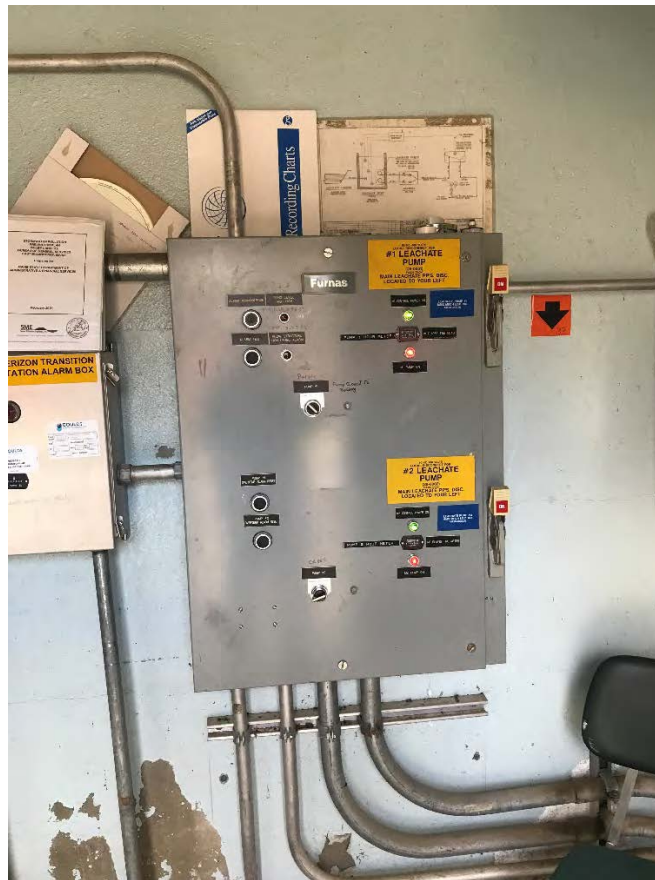
Dolby Leachate Pond Pump Control Panel
