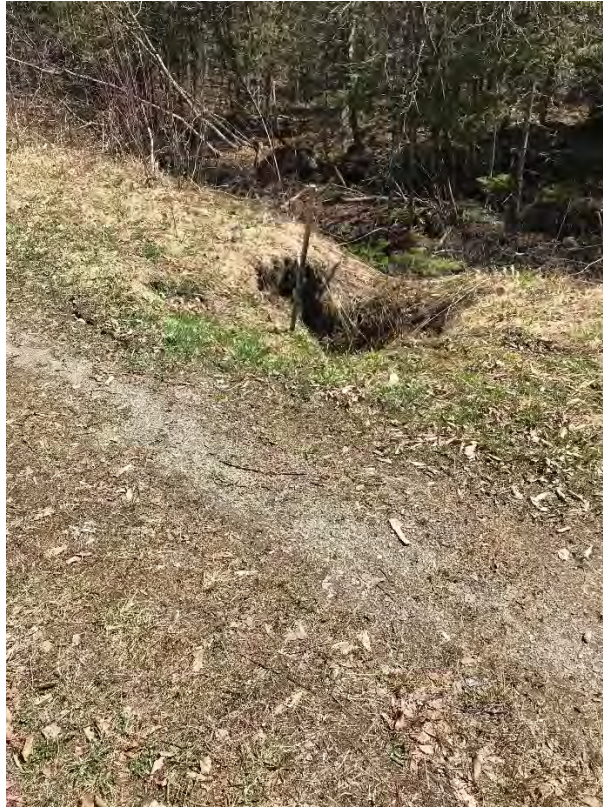
Leachate Pipeline Access Road Culvert Failure
