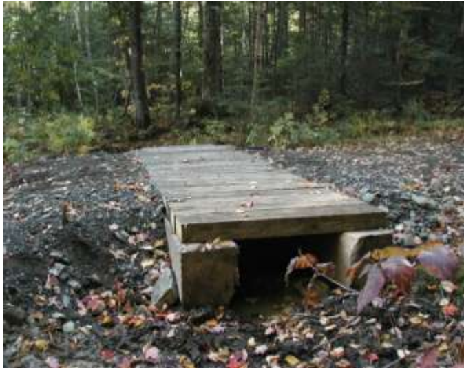
Box culvert: no gravel cover
